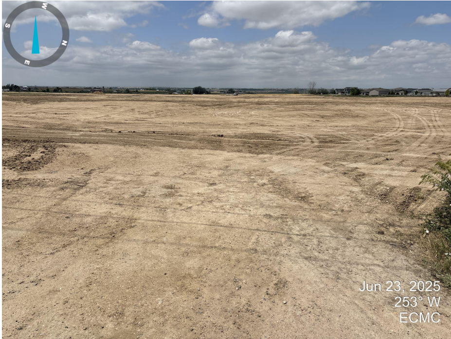
Photo 5. Looking west down the access road. The access road is within construction disturbance. The entrance ins being used for construction access.
