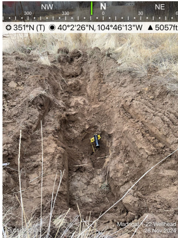
Flowline Sample Location 01
