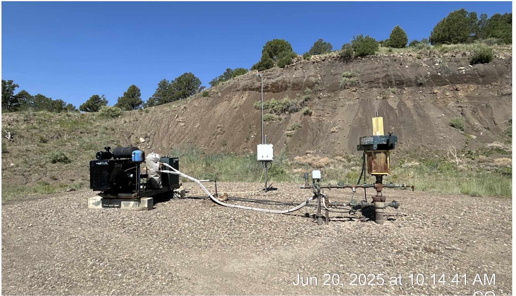
PHOTO 3: WELLHEAD AND EQUIPMENT
