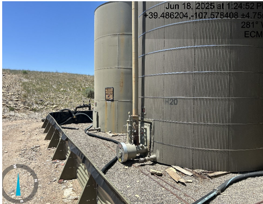
Tank signage is weathered
