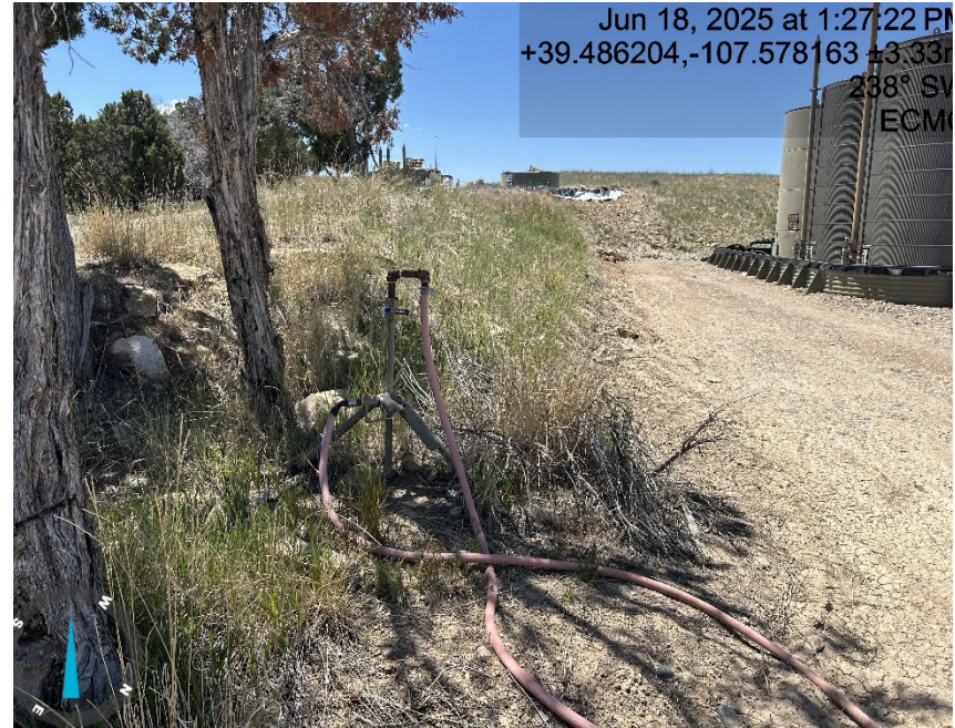
Methanol line from tank up the hill, pump handle zip tied open, 1 inch ball valve closed. No evidence of containment in case of spill.
