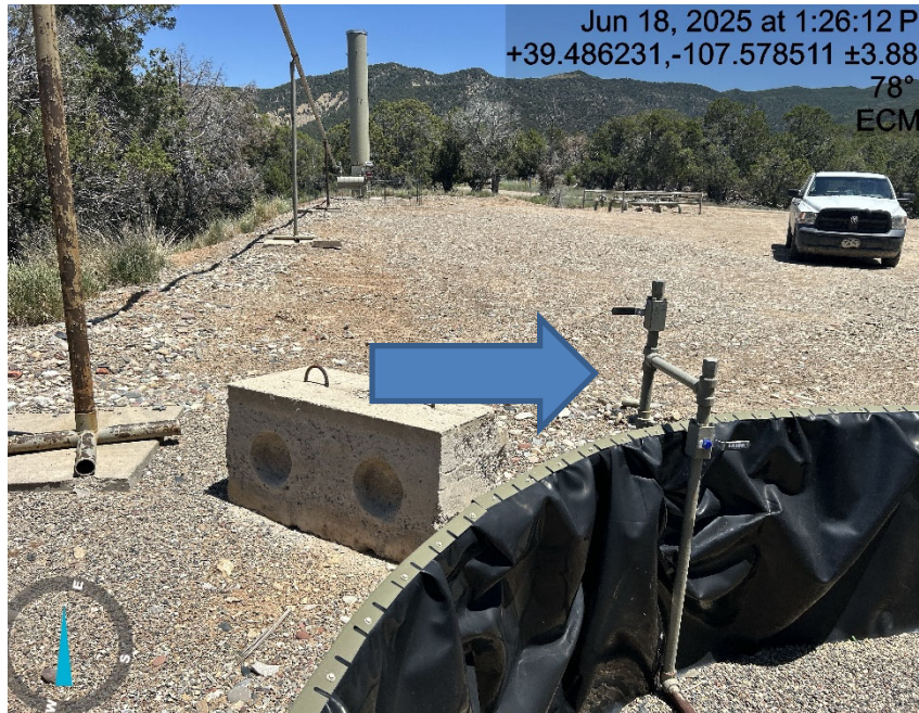
Supply gas to ECD is connected at tank battery
