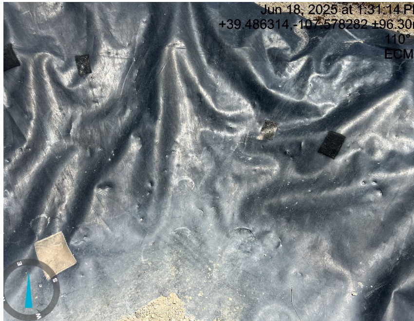
Holes in liner at methanol tank
