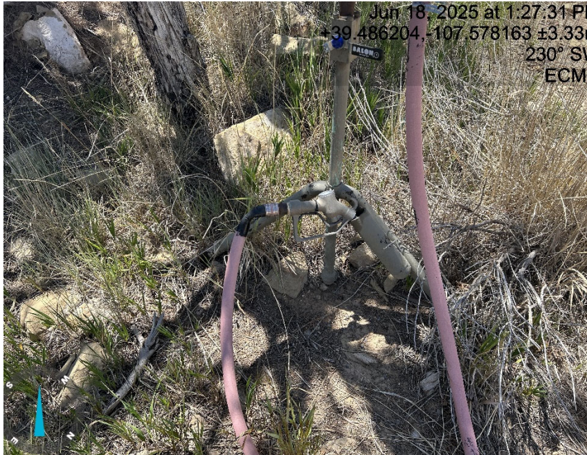
Methanol line from tank up the hill, pump handle zip tied open, 1 inch ball valve closed. No evidence of containment in case of spill.
