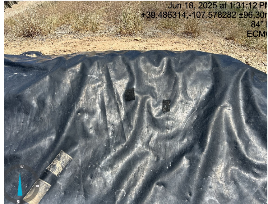
Holes in liner at methanol tank
