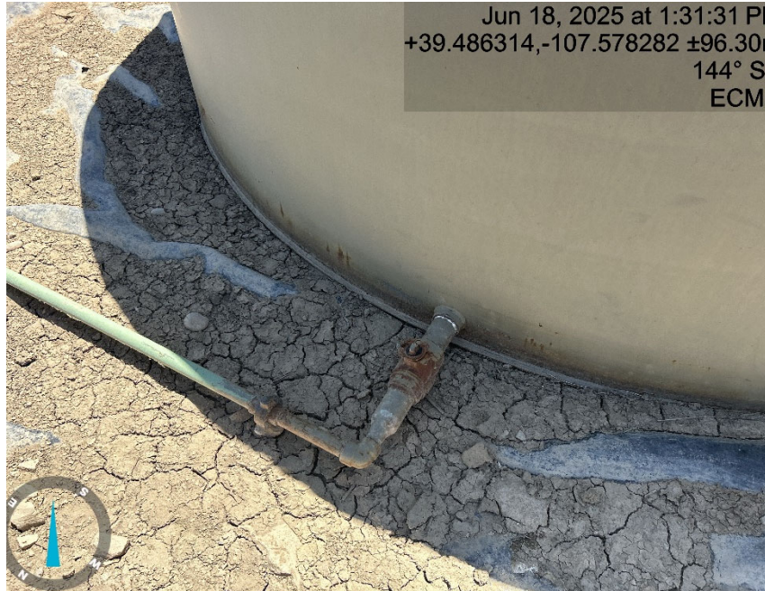
Methanol tank ball valve open
