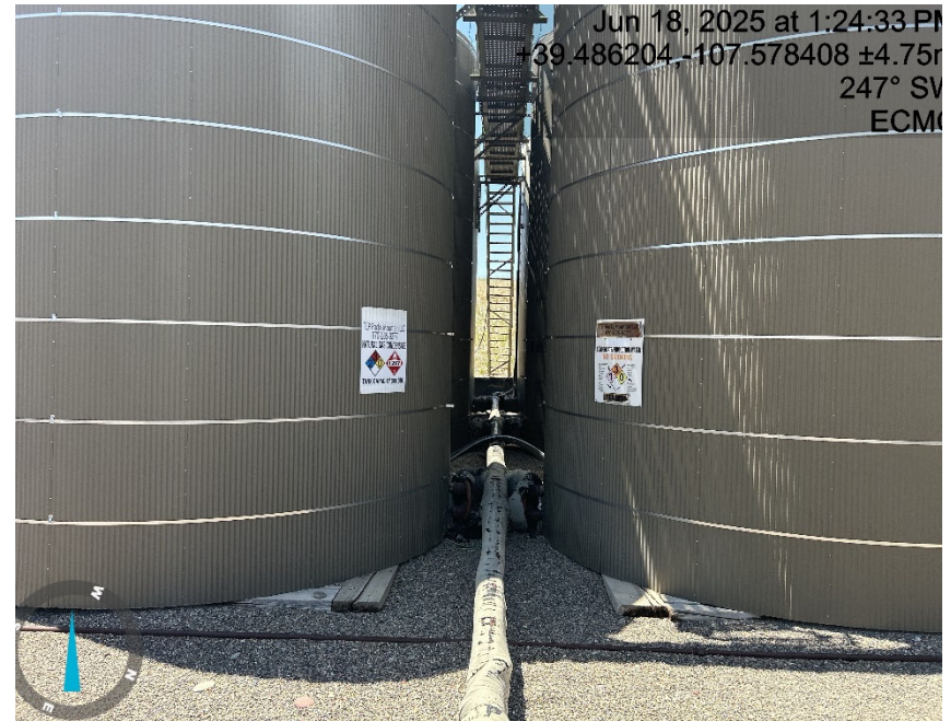
Tank signage is weathered
