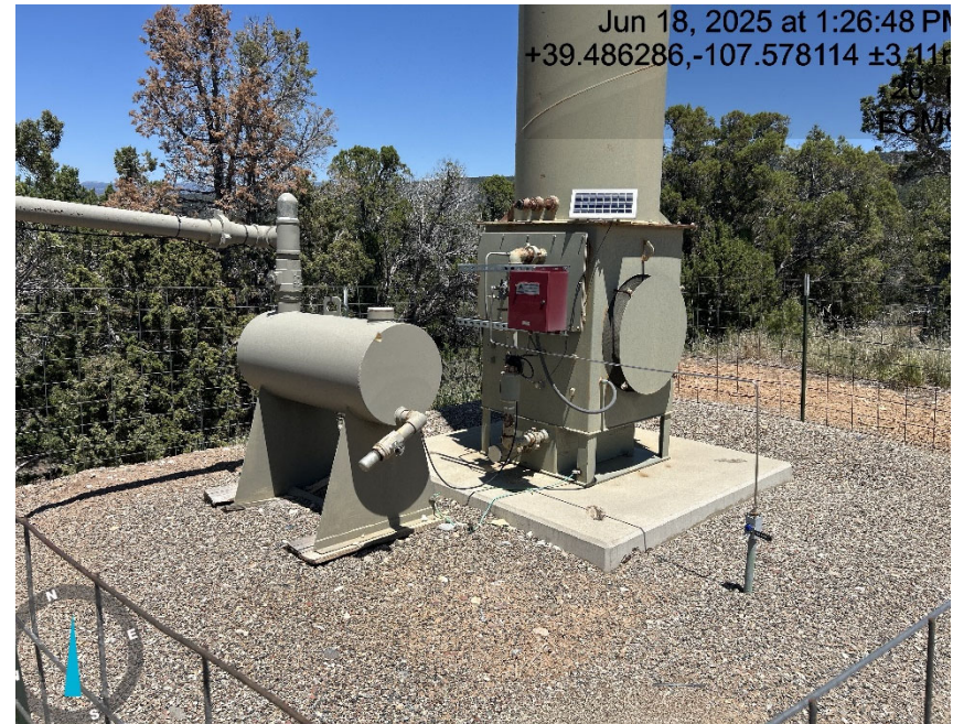
Supply gas is connected at ECD pilot is not running, main line from tanks is disconnected and not metered
