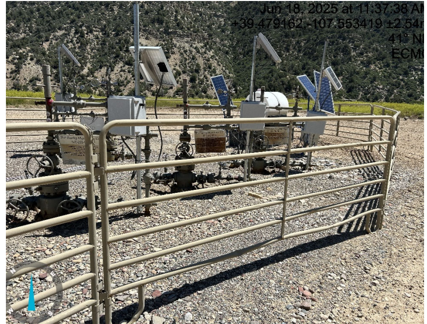
Well signage is illegible
