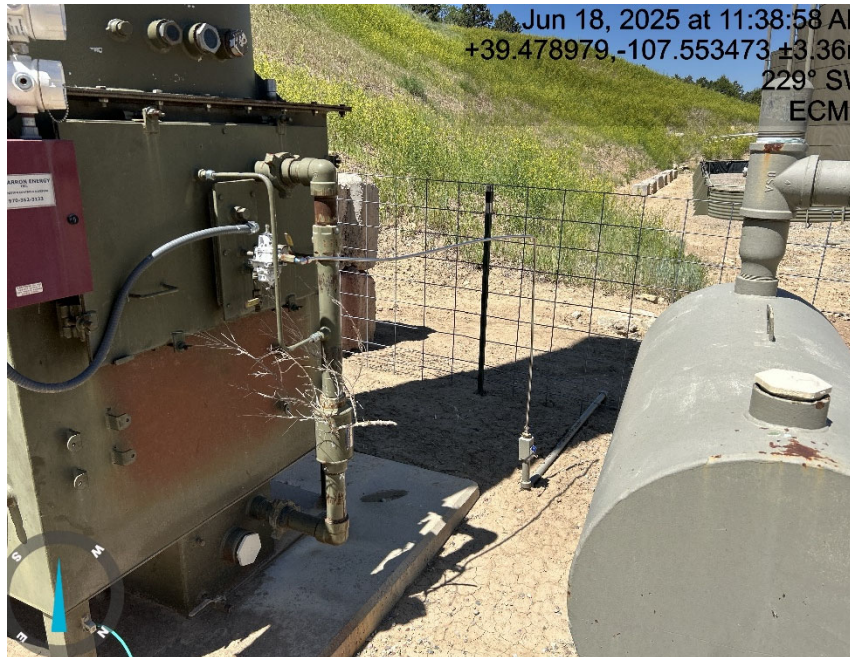
ECD supply gas is connected valve shut and not running
