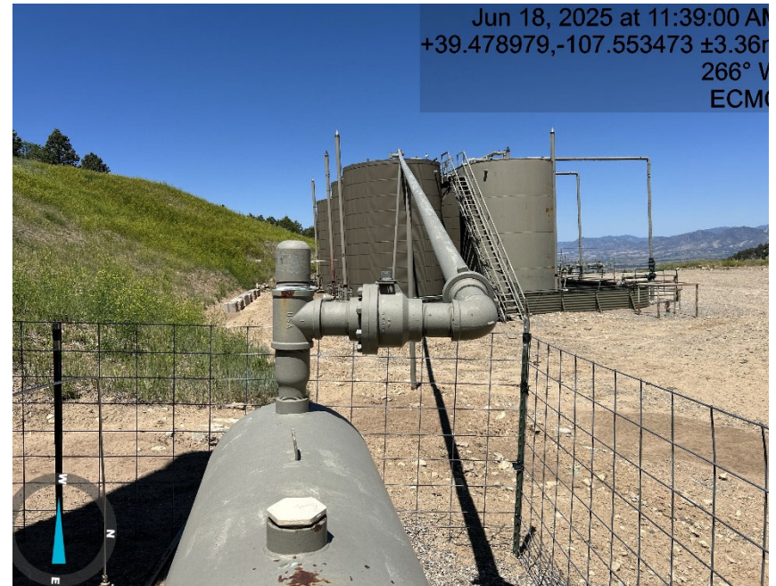
Main line from tanks is disconnected from ECD and not metered
