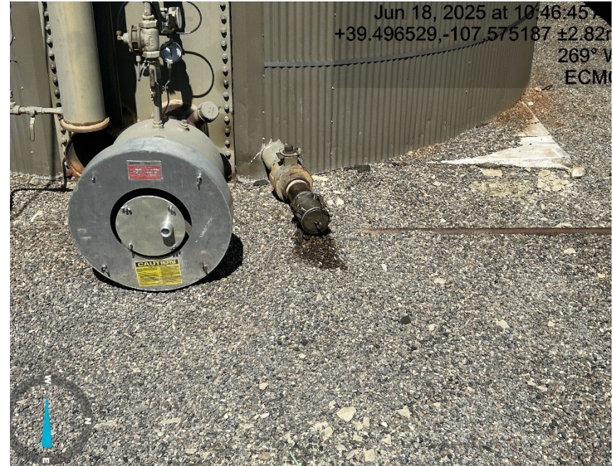
Staining under valves
