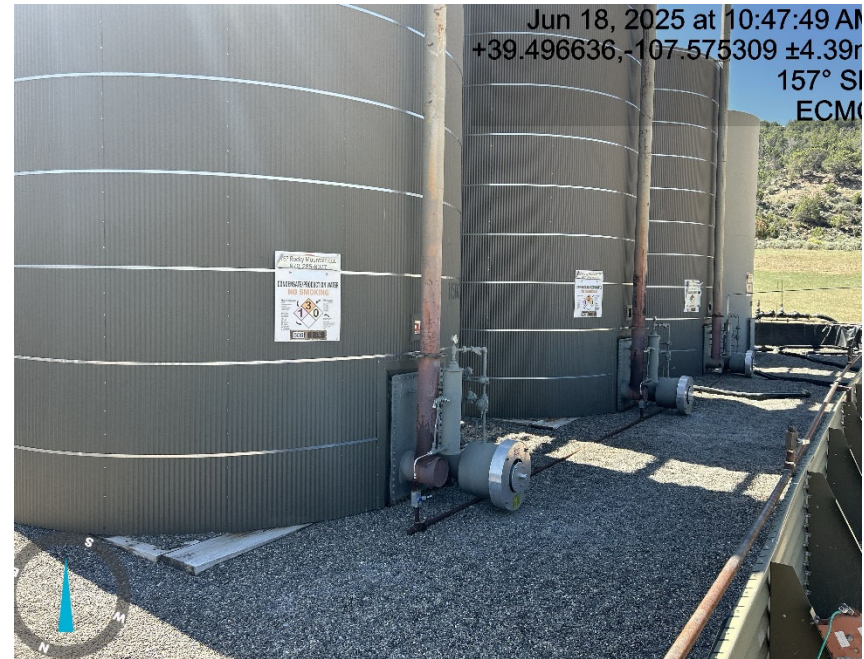
Tank labels weathered
