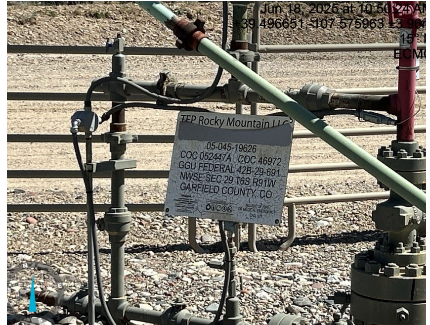
Well signs not maintained
