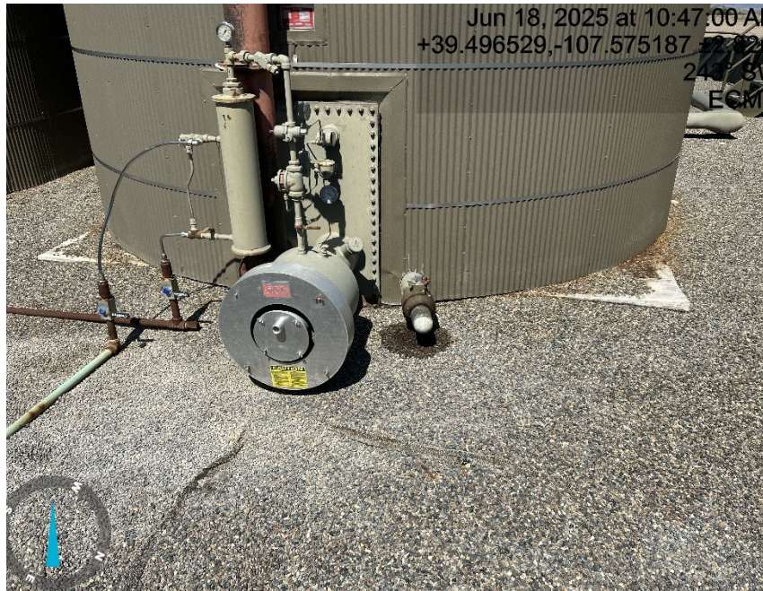
Staining under valves
