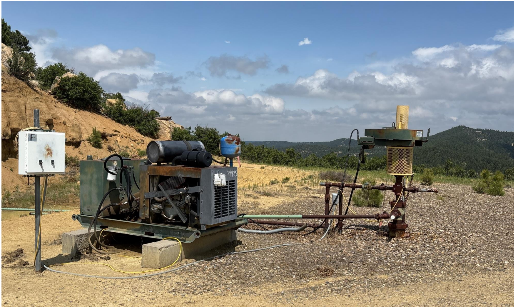
PHOTO 3: WELLHEAD AND EQUIPMENT.
