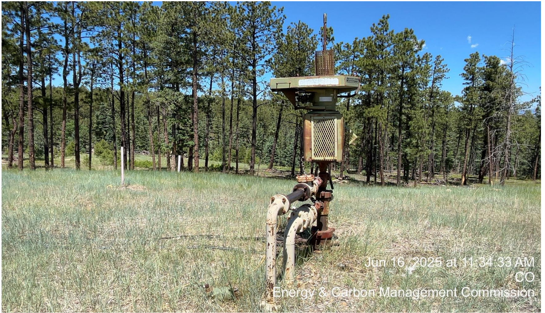
PHOTO 3: WELLHEAD AND EQUIPMENT
