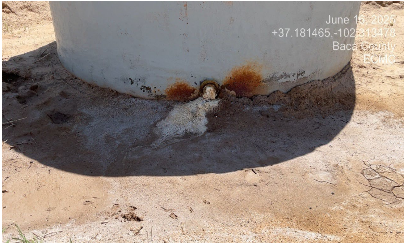
Photo 2. There is a leak at the tank which needs to be repaired. New tank may be needed.
