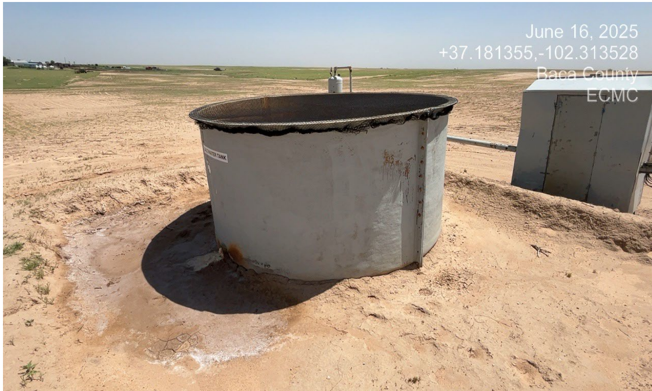
Photo 2. The netting on the tank has been repaired and maintained. There is a leak that occurred which was contained in the secondary containment.
