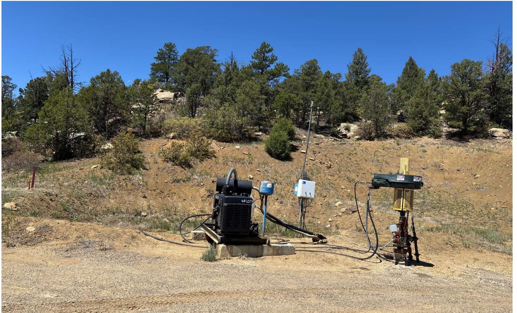
PHOTO 3: WELLHEAD AND EQUIPMENT.
