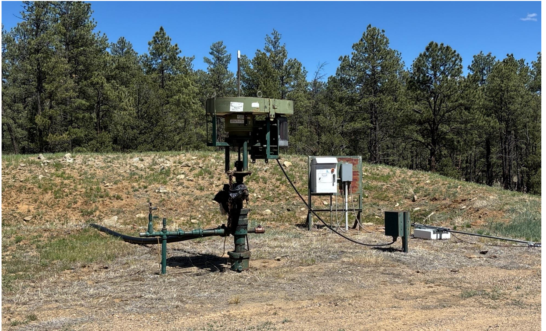
PHOTO 4: WELLHEAD AND EQUIPMENT.
