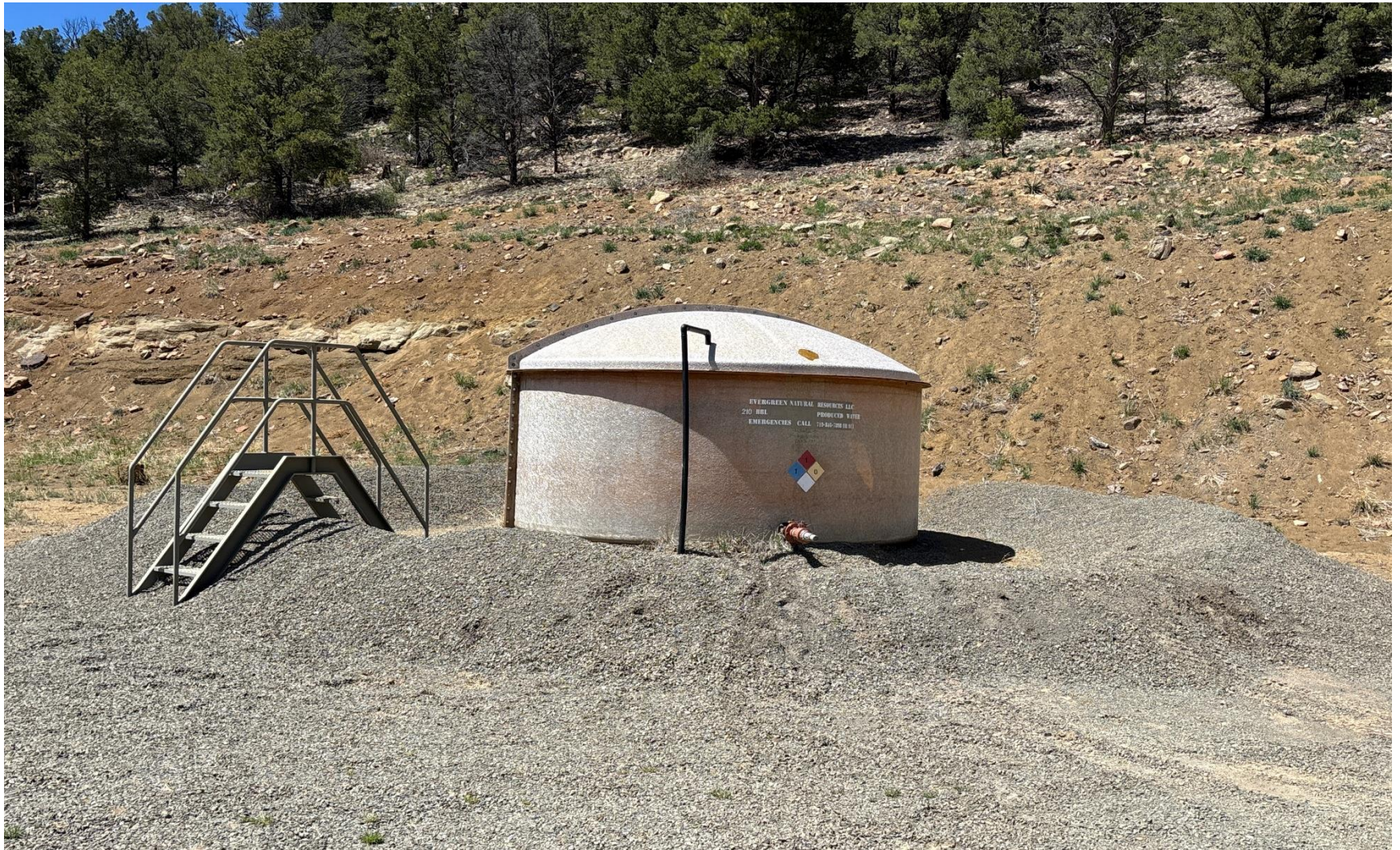
PHOTO 4: PRODUCED WATER TANK BATTERY.
