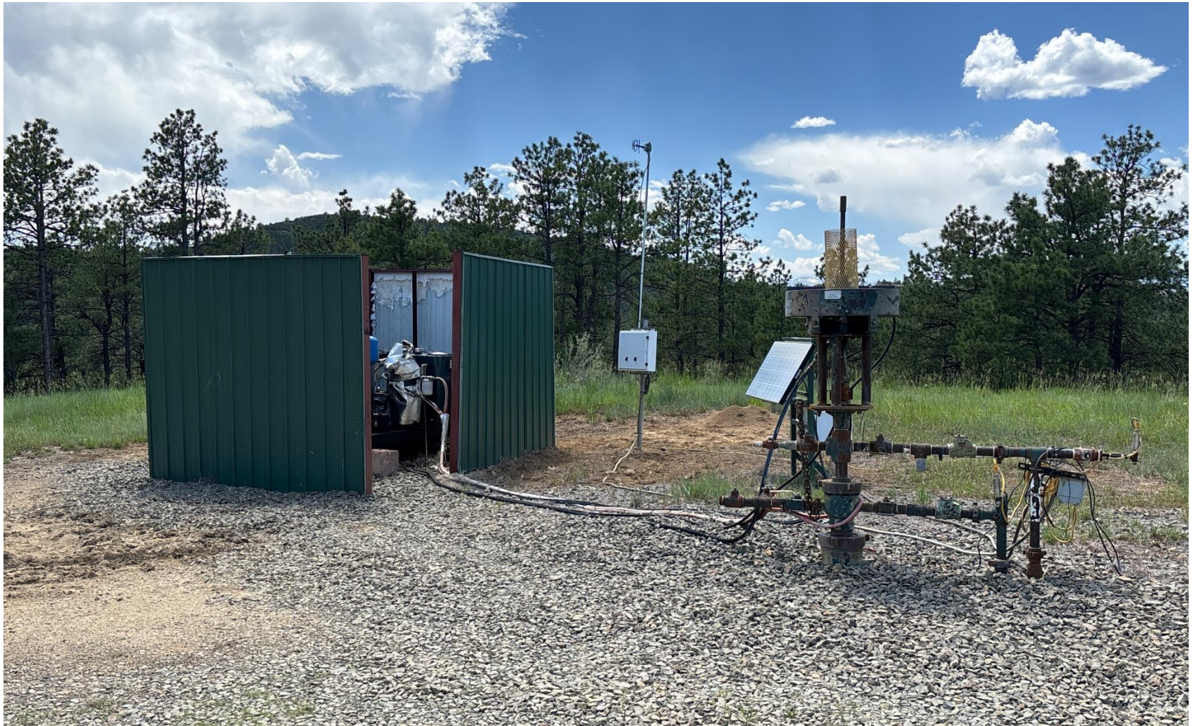
PHOTO 3: WELLHEAD AND EQUIPMENT.
