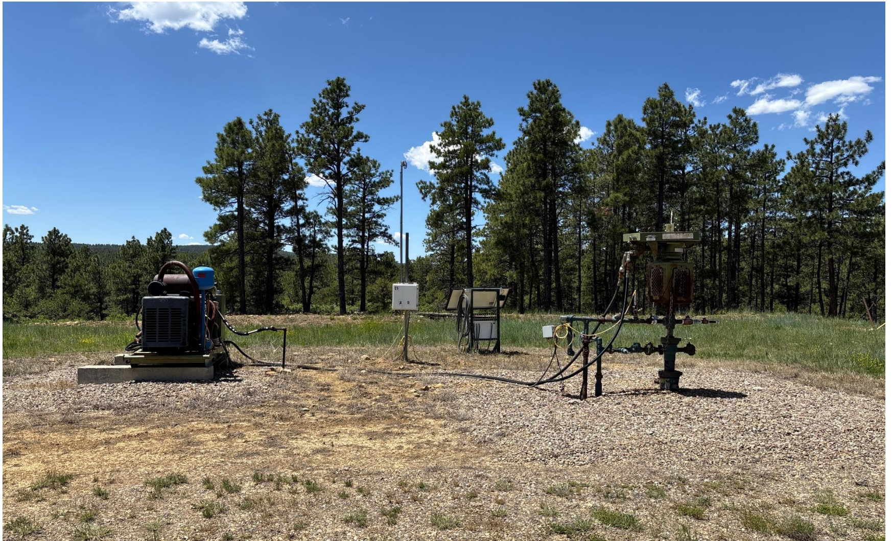
PHOTO 3: WELLHEAD AND EQUIPMENT.
