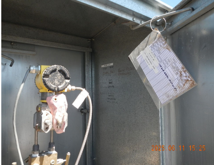
3. Gas Meter inside Meter Box.
