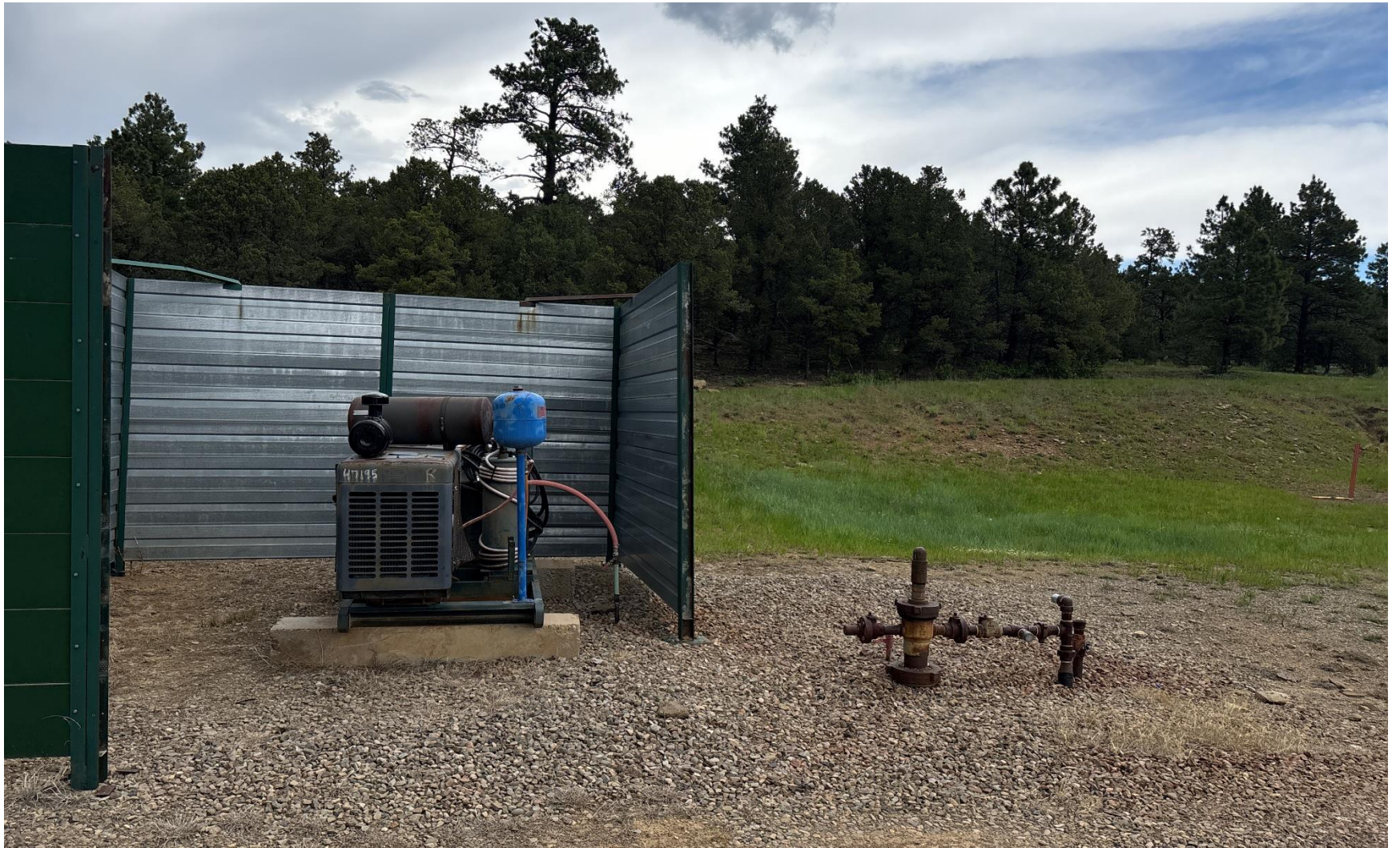
PHOTO 3: WELLHEAD AND EQUIPMENT.
