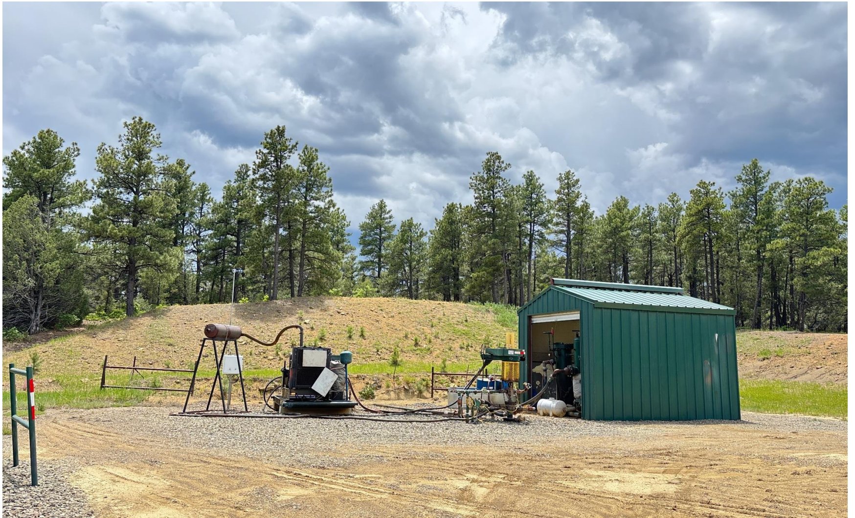
PHOTO 3: WELLHEAD AND EQUIPMENT.
