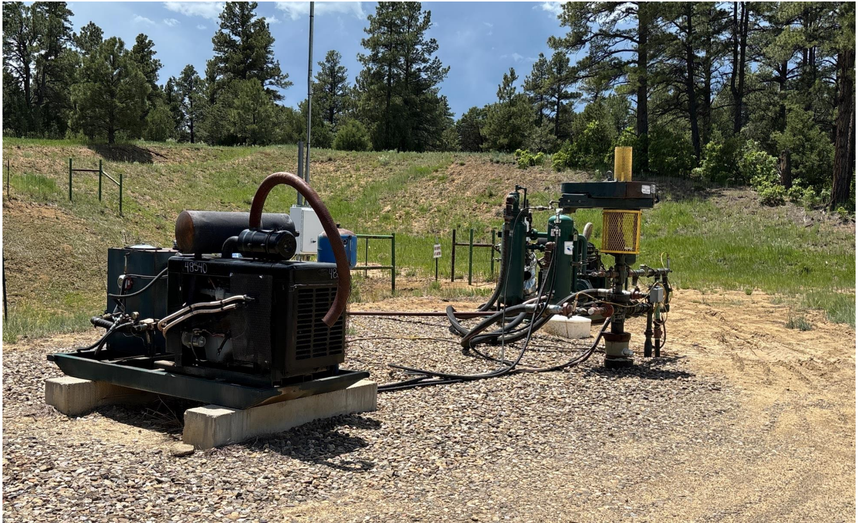
PHOTO 3: WELLHEAD AND EQUIPMENT.
