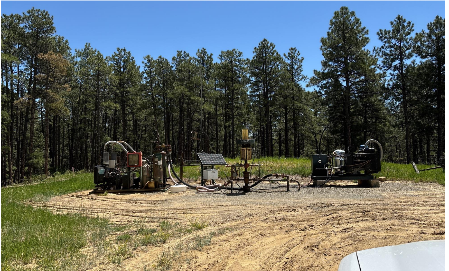
PHOTO 3: WELLHEAD AND EQUIPMENT.
