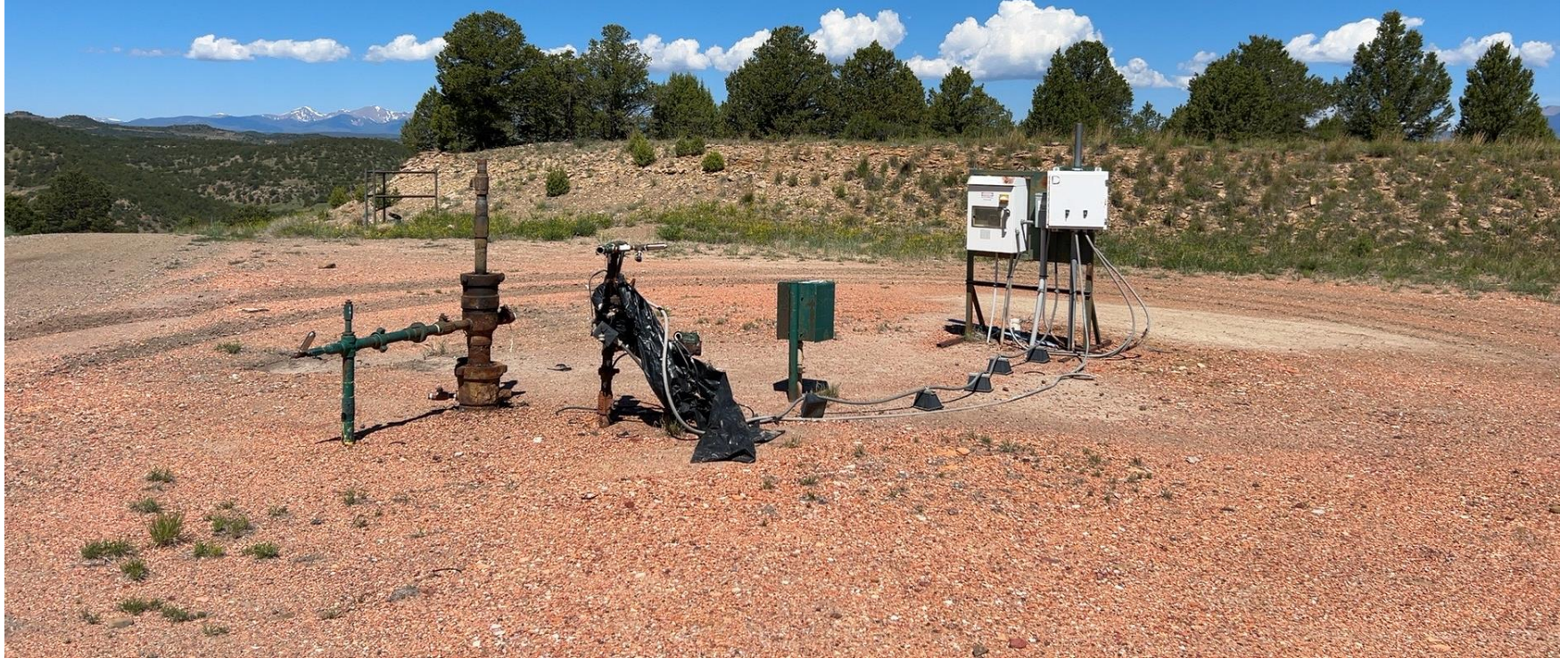
PHOTO 3: WELLHEAD AND EQUIPMENT
