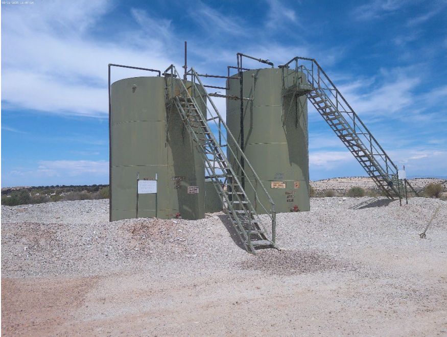
Tank Battery for producing well
