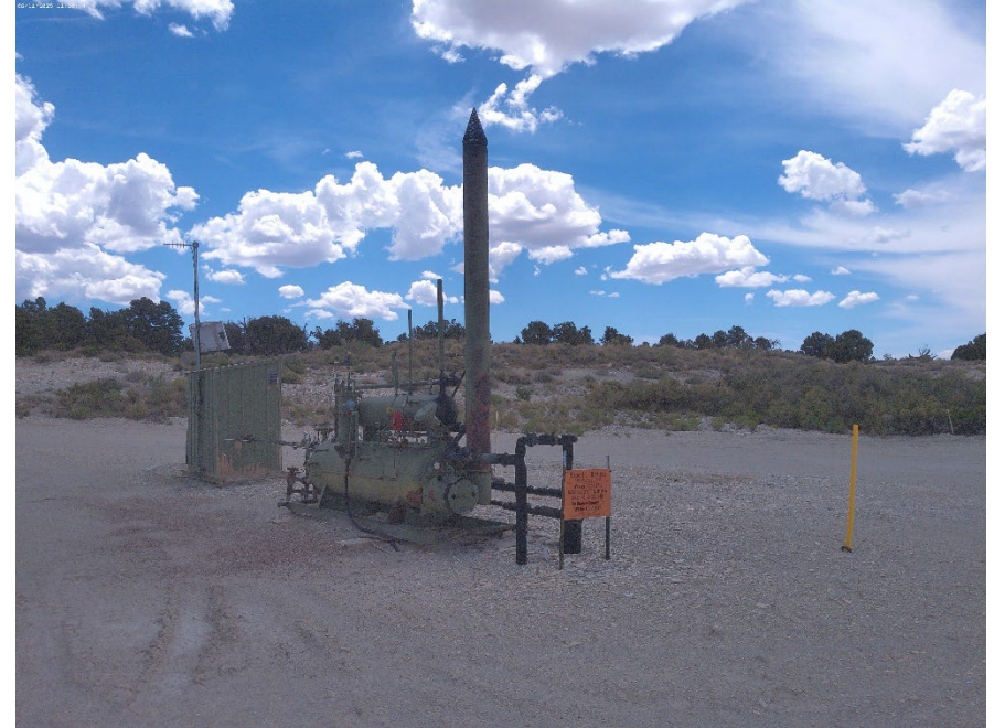
Separator and Meter Housing
