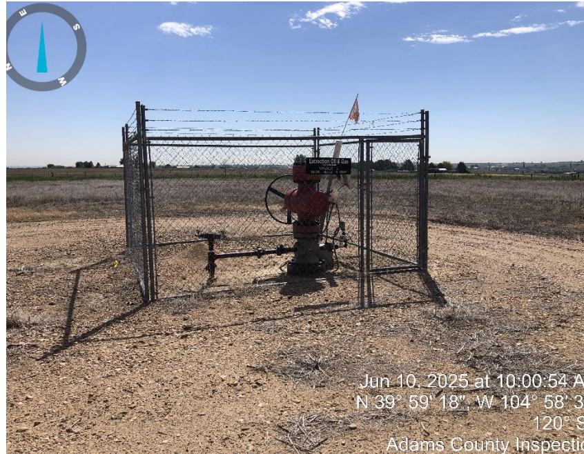
Photo #3 Well head.
