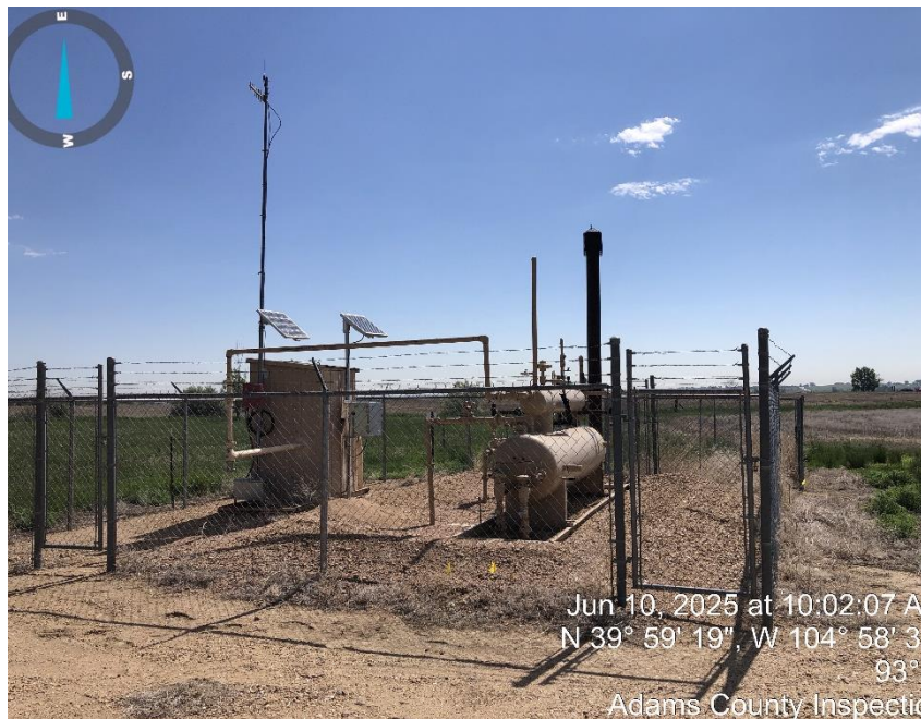
Photo #2 Meter house & separator.
