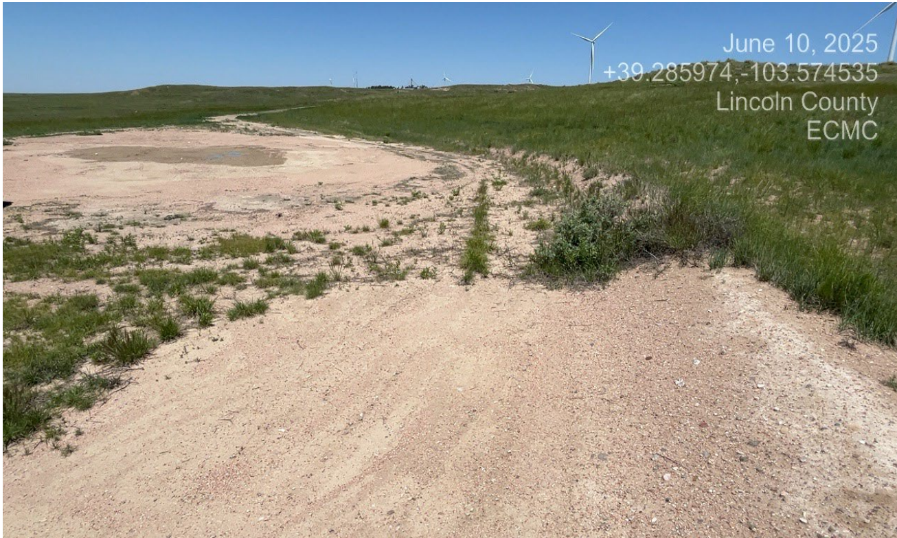
Photo 4. Facing orthwest at the location. Gravel has not been removed and soils are not decompacted and regraded.
