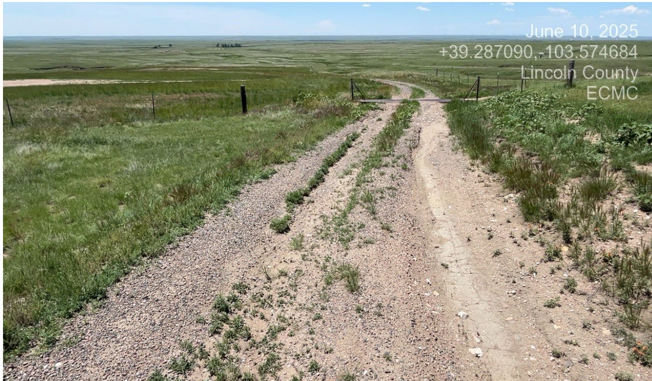
Photo 2. Facing south further down the road. There is erosion at this area of the road. The cattleguard will need to be removed.
