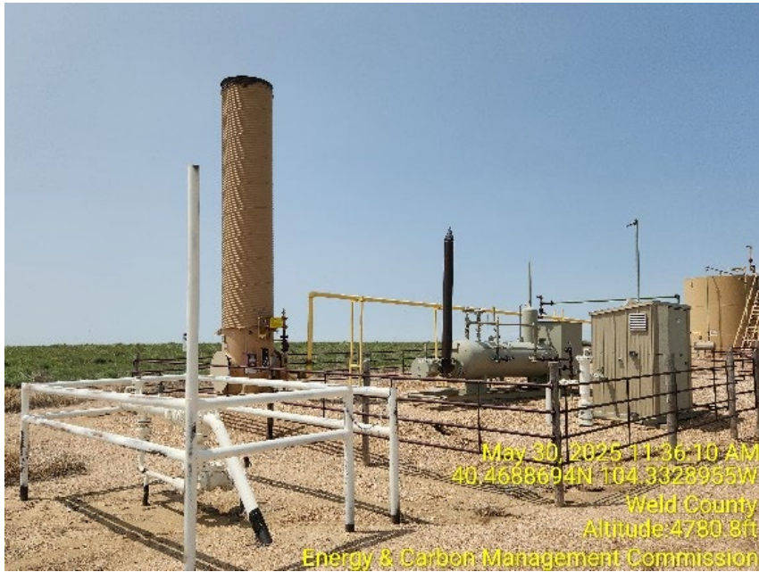
Photo 3 – ECD, Separator and Gas Meter
