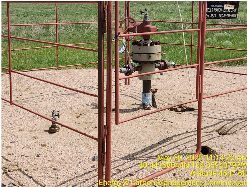
Photo 3 – Tank Battery - Tumbleweed
