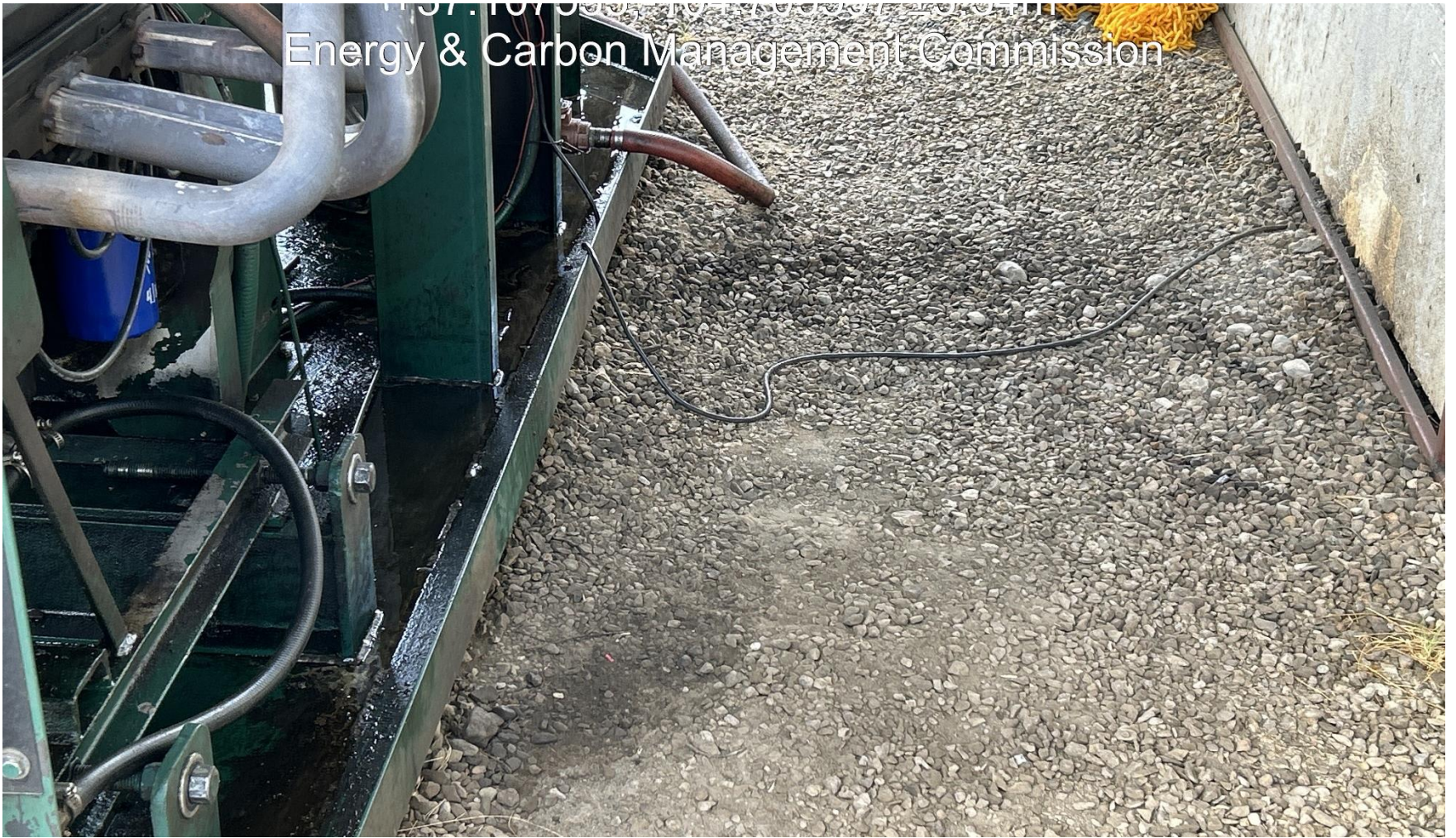
PHOTO 4: Stained soil around ring
