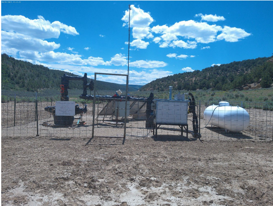
Injection wellhead with line heater and Telemetry
