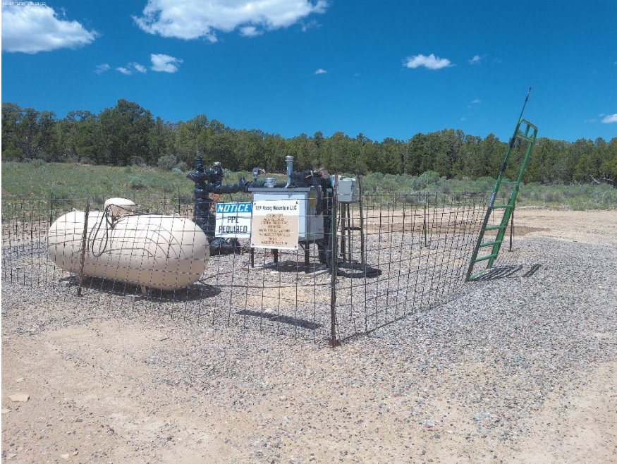
Injection wellhead and line heater
