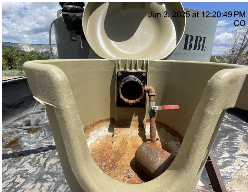
Photo # 5830 Open ended load line
