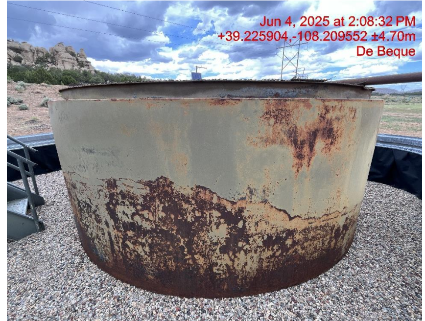
Photo # 7739 Tank is dented, also rusted in most areas
