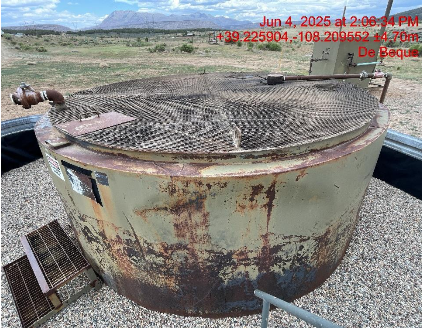
Photo # 7733 Tank is dented, also rusted in most areas
