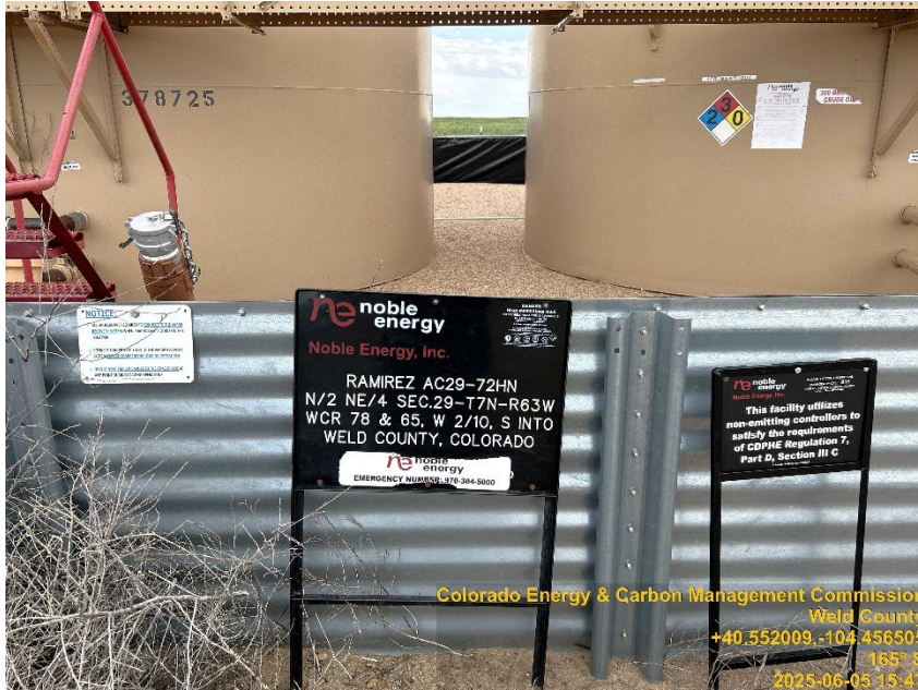
Photo #3 Ramirez AC 29-72HN Battery site Active Battery signage
