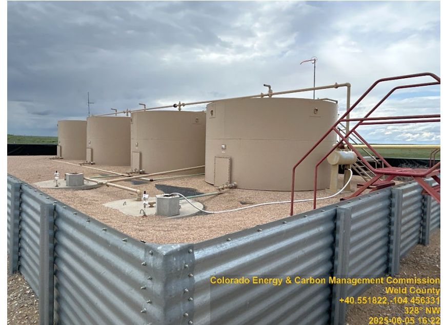
Photo #4 Ramirez AC 29-72HN Battery site Active Crude oil, produced H2O tank(s): SE corner
