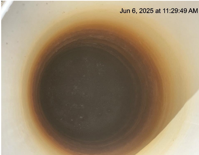
Photo # 7214 UNOCAL 24-9DRD leak
