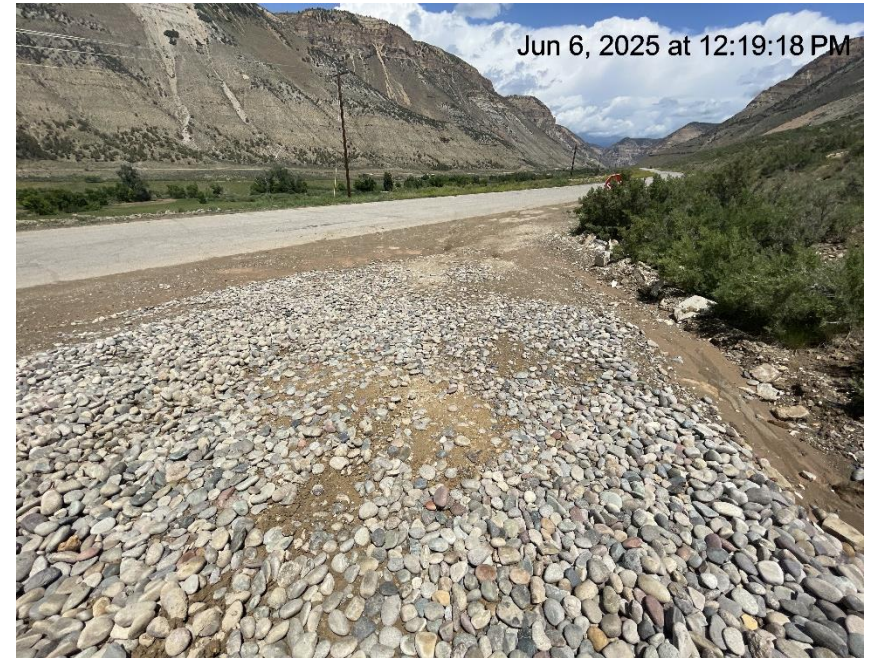
Photo # 7236 Tracking pad/BMP at intersection of CR 215 & start of lease road has not been improved
