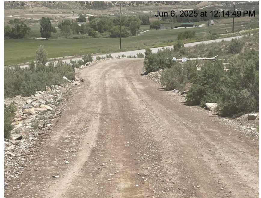
Photo # 7234 BMP's have not been added to stabilize the lease road
