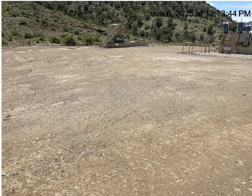
Photo # 7229 BMP's have not been added to stabilize the working surface of the pad
