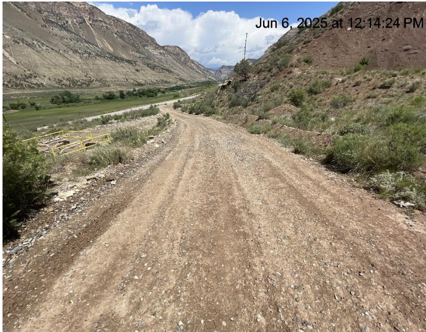
Photo # 7233 BMP's have not been added to stabilize the lease road
