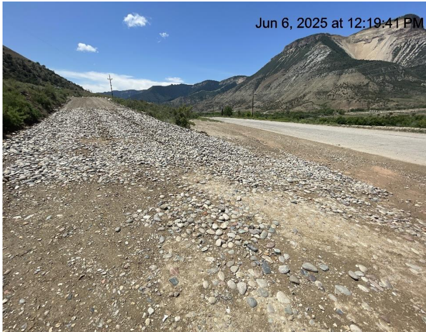
Photo # 7237 Tracking pad/BMP at intersection of CR 215 & start of lease road has not been improved
