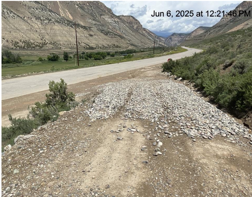
Photo # 7235 Tracking pad/BMP at intersection of CR 215 & start of lease road has not been improved
