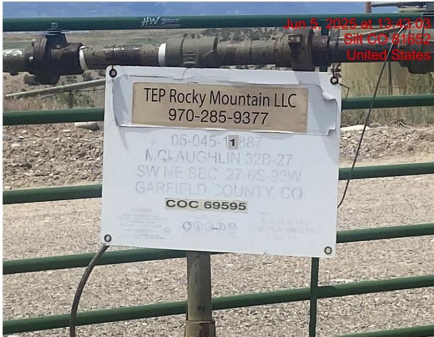
Illegible Wellhead Sign – Photo #09149
