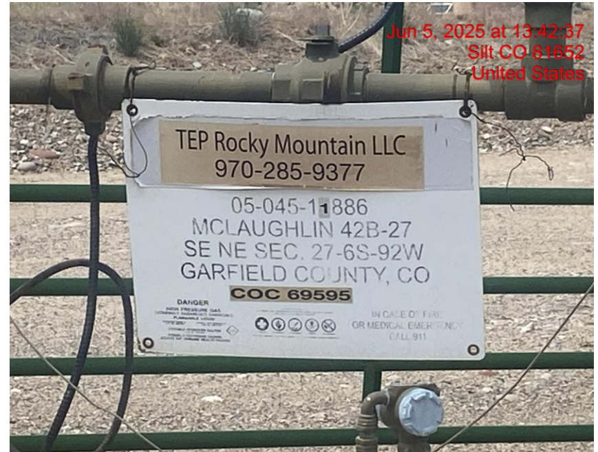
Illegible Wellhead Sign – Photo #09146
