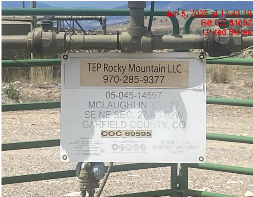
Illegible Wellhead Sign – Photo #09151
