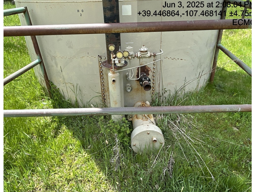
Recent inspection C/A still present
