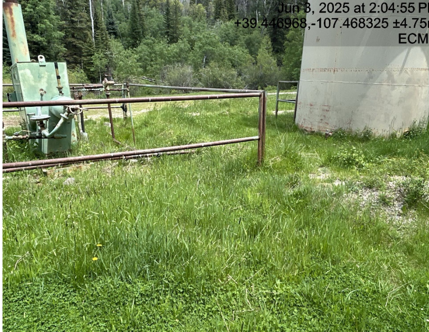
Insufficient containment and weeds
