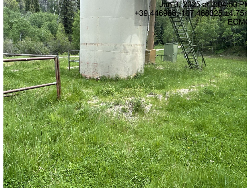
Insufficient containment and weeds
