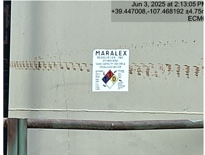
Recent inspection C/A still present
