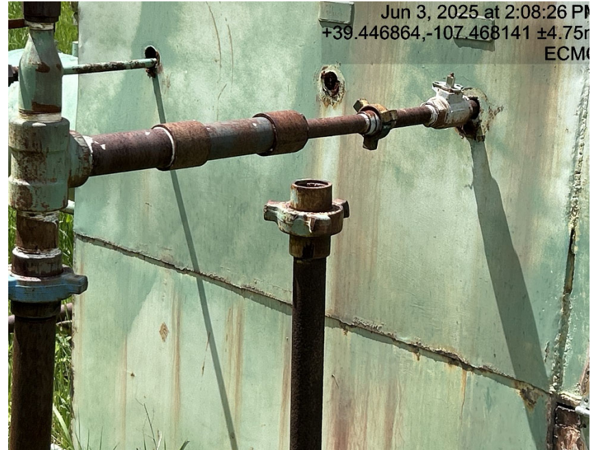
Recent inspection C/A still present
