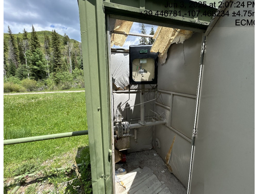
Recent inspection C/A still present
