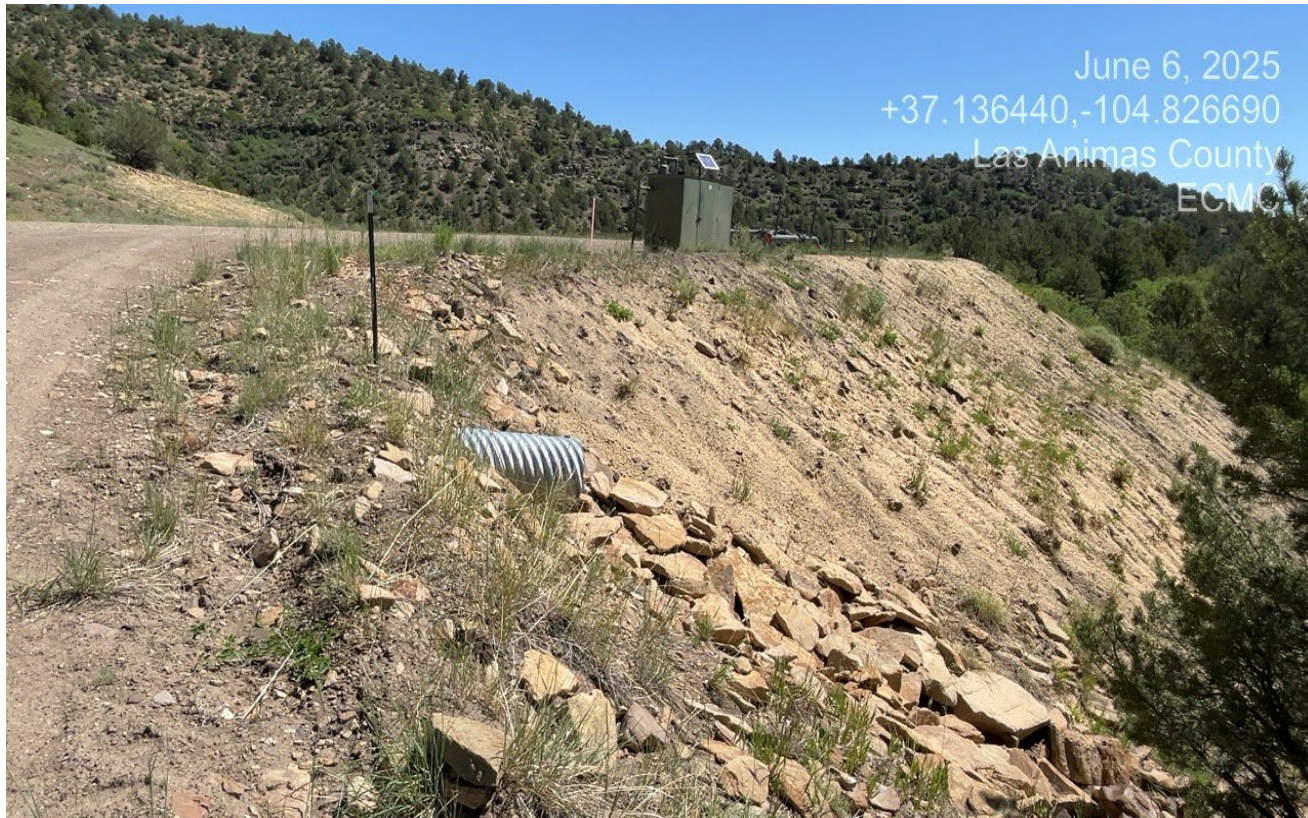
Photo 5. Facing east toward the fill slope which has been seeded and hydromulched.
