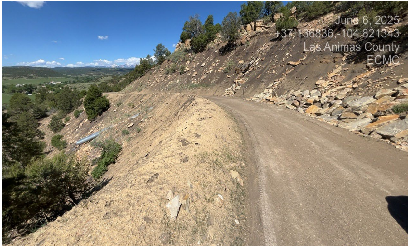
Photo 1. Facing west along the access road. The erosion along the road has been repaired and stabilized.
