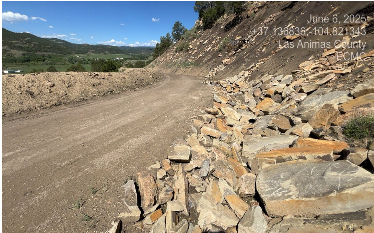
Photo 2. Facing southwest along the access road. There is rp/rap placed along the roadside where erosion was occurring.
