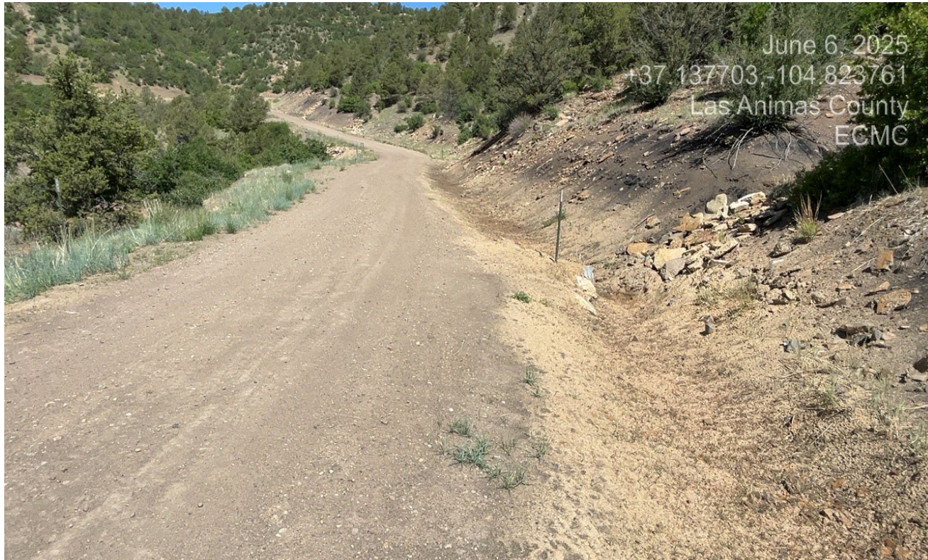
Photo 3. Facing west along the access road. The culverts and ditches along the road have been cleaned out.
