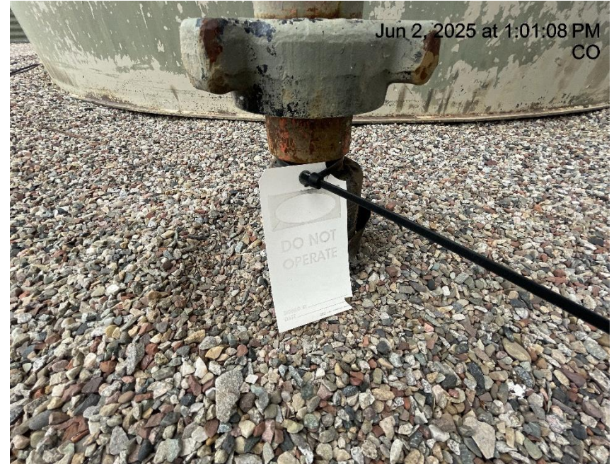
Photo # 6008 Tag on unused flowline faded & becoming illegible
