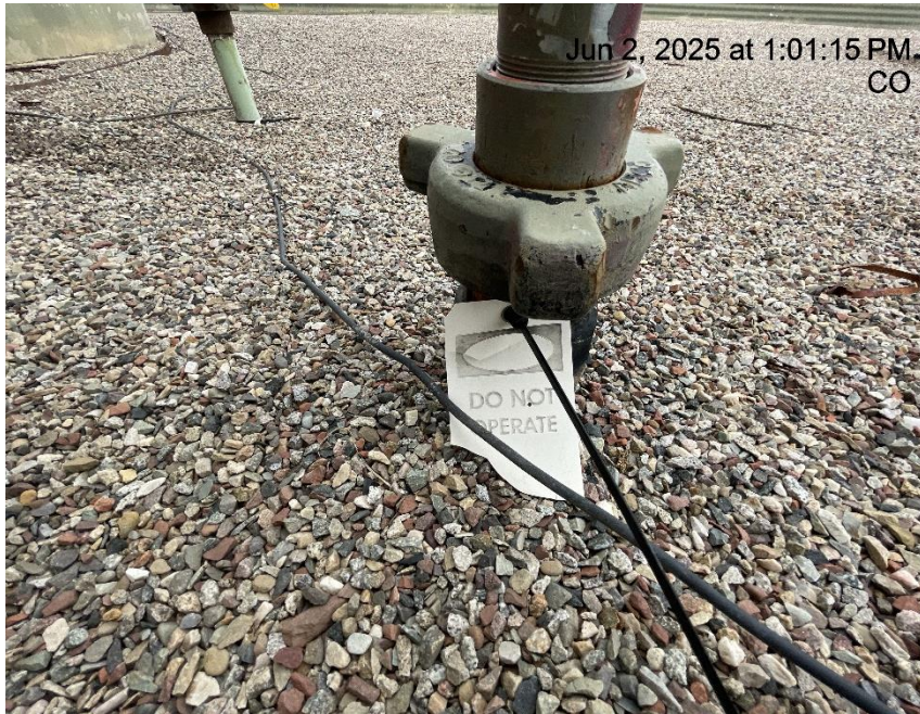
Photo # 6009 Tag on unused flowline faded & becoming illegible
