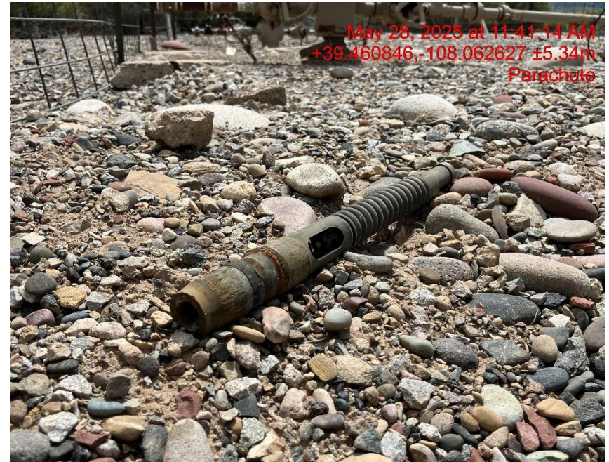
Photo # 7435 Debris near wellheads
