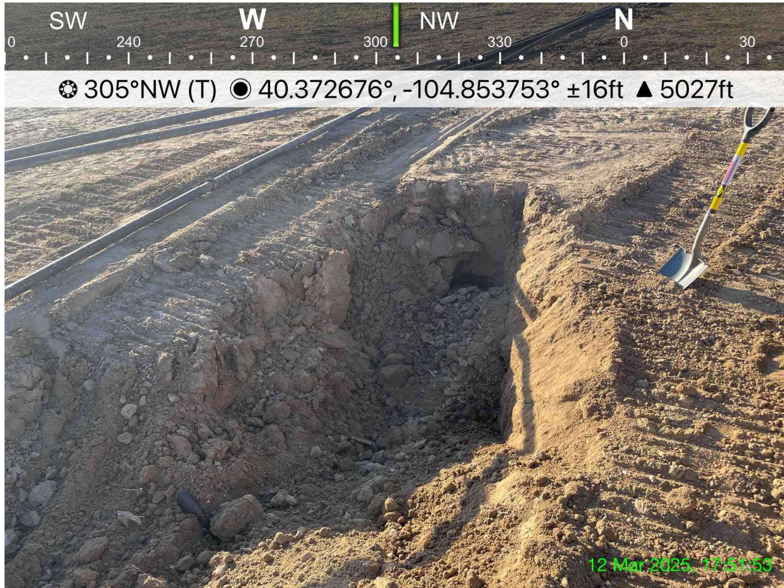
Photo 17: View of sampling location FL01-R-W, facing northwest
