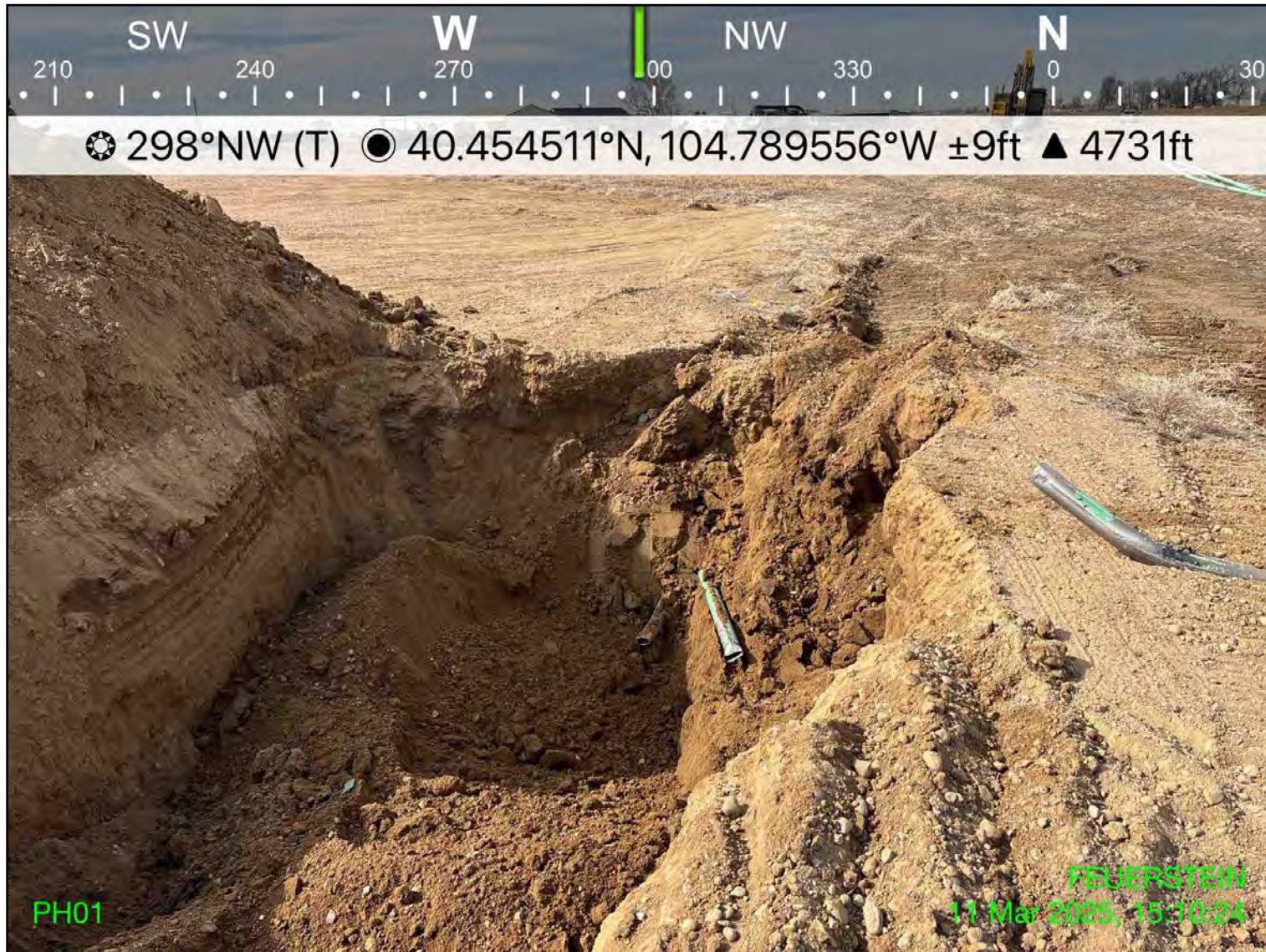
Photo 4: View of pothole location 1, facing northwest
