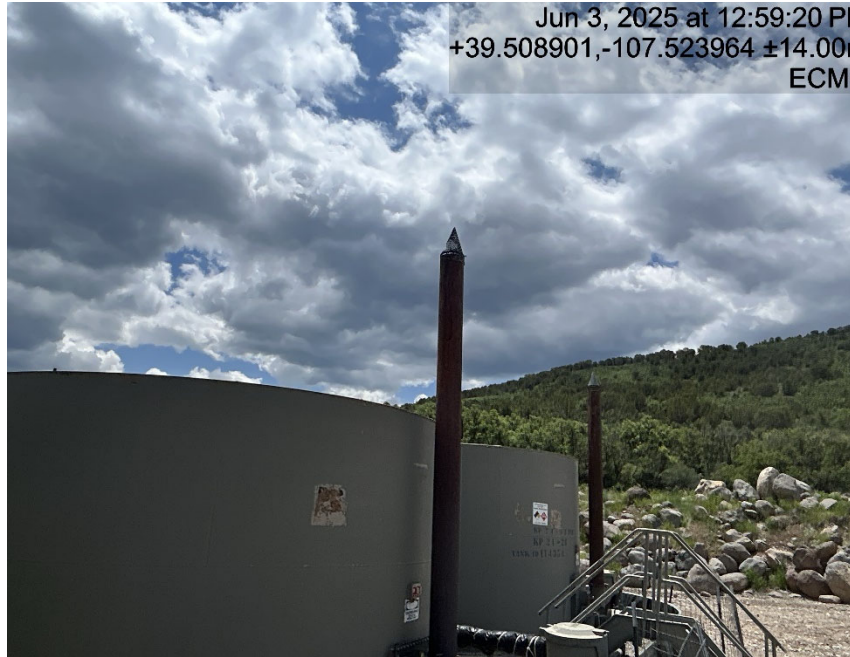
Failing bird protector
