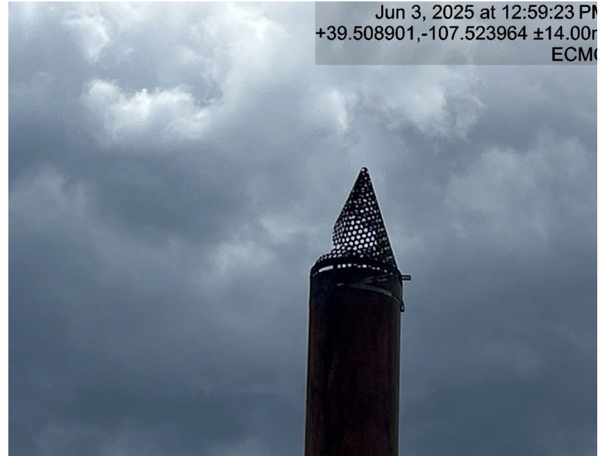
Failing bird protector
