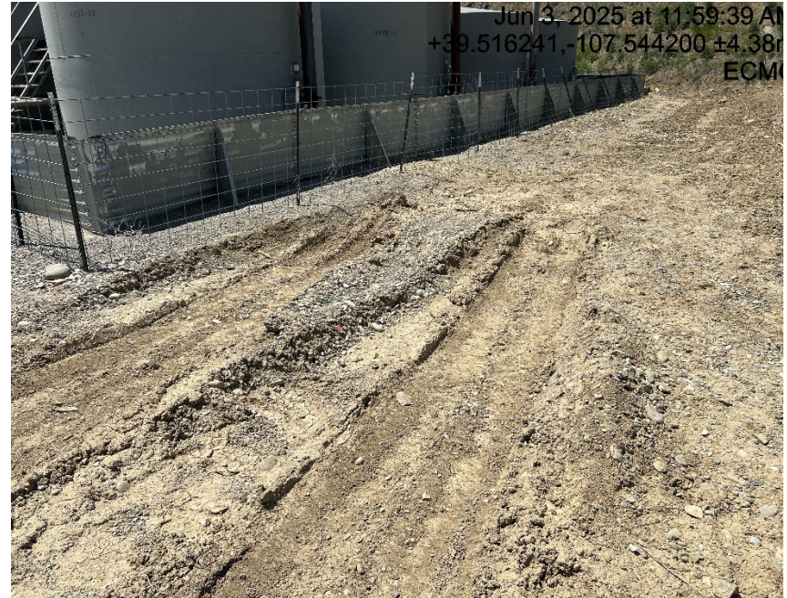
Lack of stabilization/compaction
