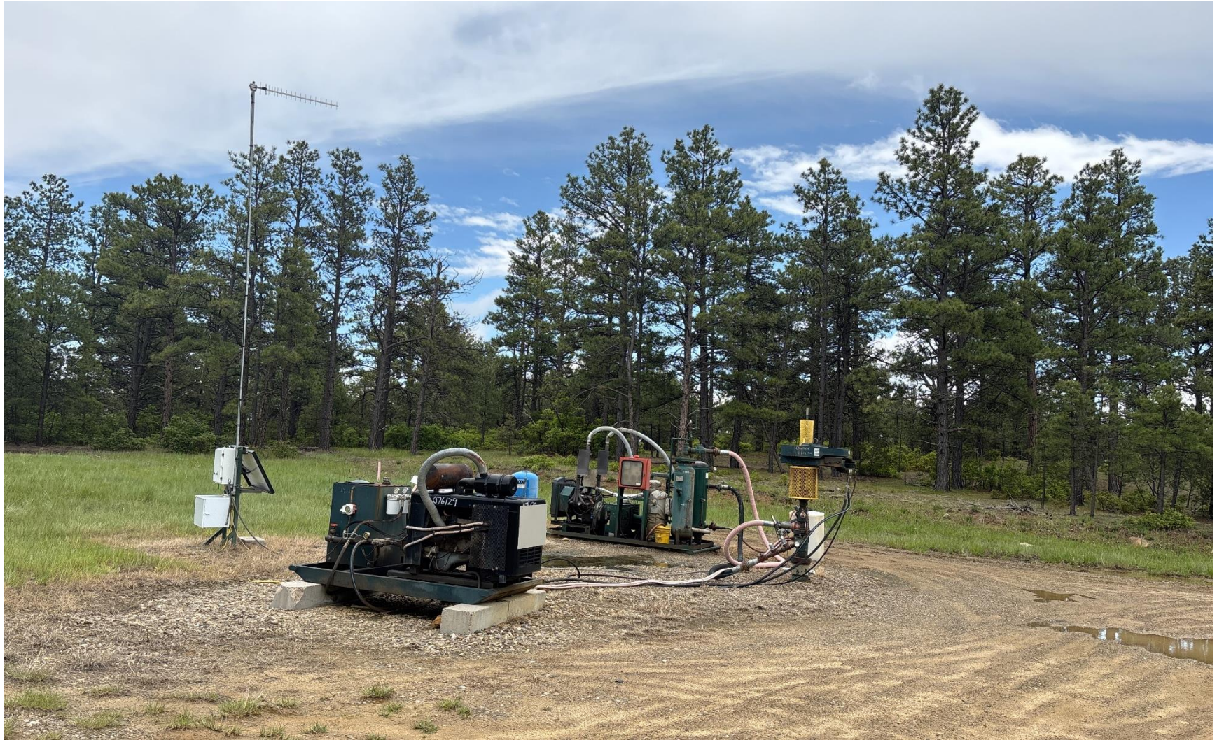
PHOTO 3: WELLHEAD AND EQUIPMENT.
