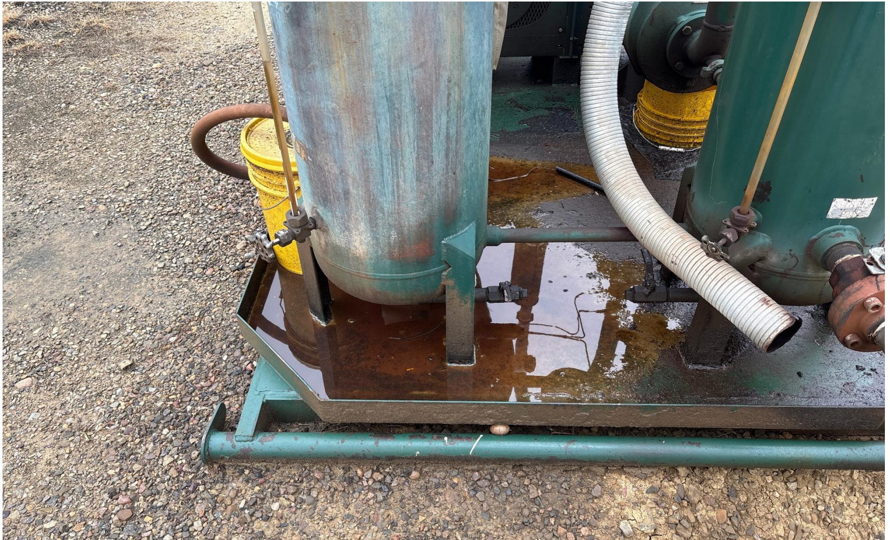
PHOTO 4: OILY WASTE IN COMPRESSOR SKID. DRAIN OILY WASTE REPAIR ALL LEAKS AND REMOVE IMPACTED SOIL PER RULE 1002..(2).D & 1002.f.(2)B, Comply with general provisions of the oil and gas act for wildlife protection AND SB-181. CA DATE 6/5/2025.
