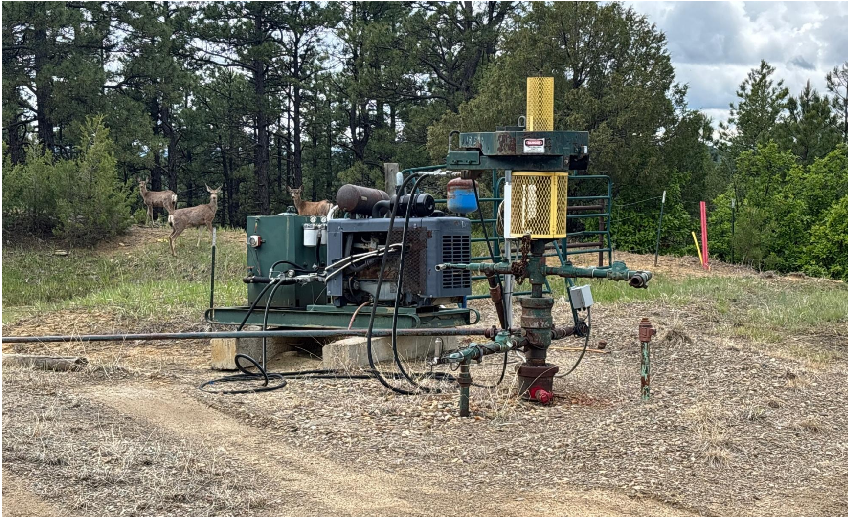
PHOTO 3: WELLHEAD AND EQUIPMENT.
