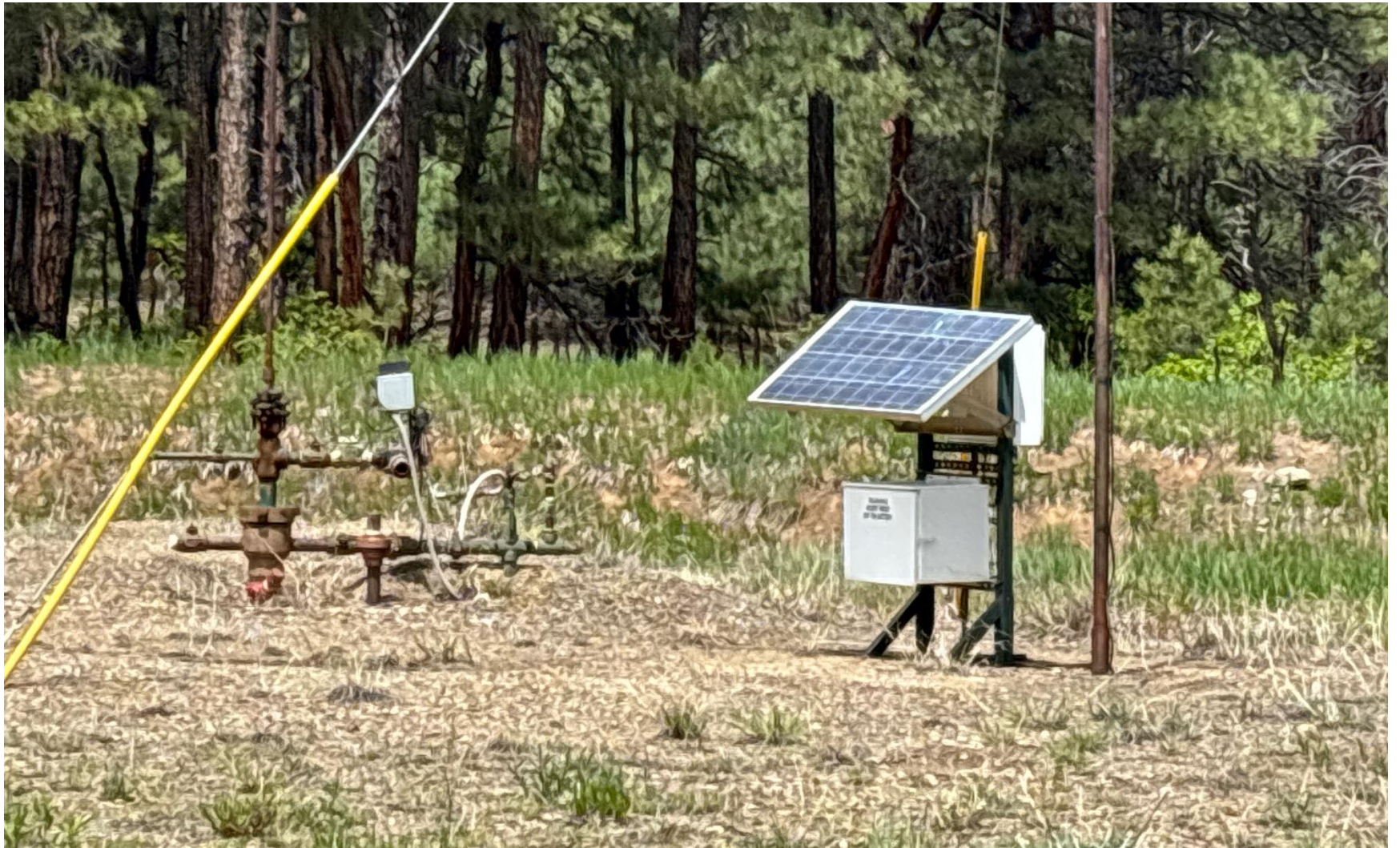
PHOTO 3: WELLHEAD AND EQUIPMENT.
