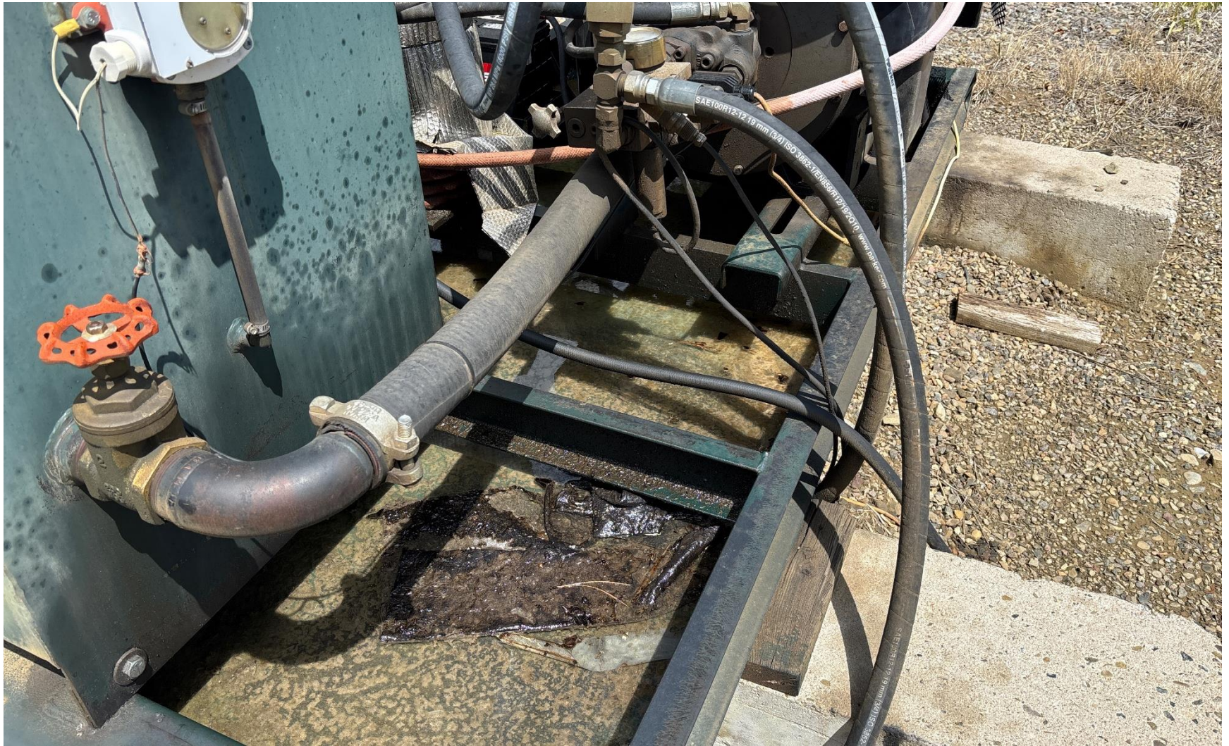
PHOTO 5: TRASH INSIDE PRIME MOVER ENGINE SKID. REMOVE TRASH PER RULE 606. CA DATE 6/10/2025.
