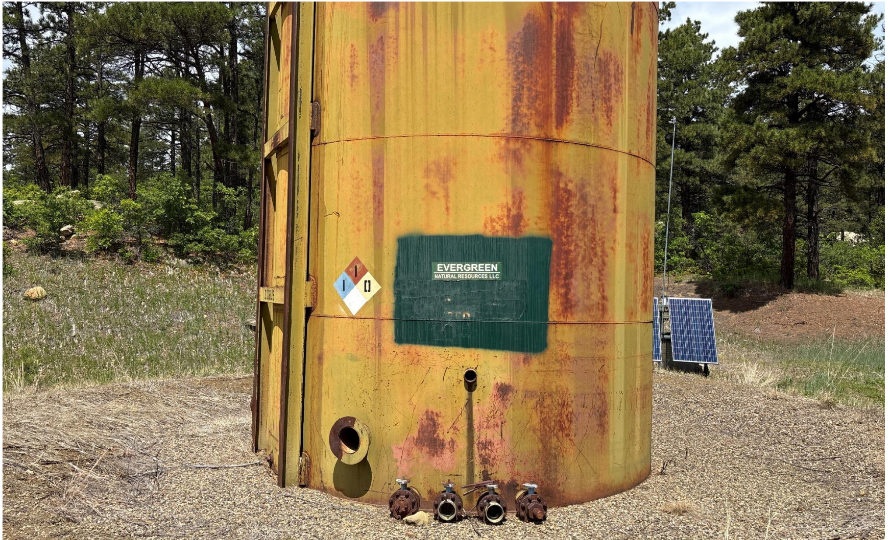
PHOTO 6: CONTENTS IS NOT LISTED ON TANK BATTERY. Install sign to comply with Rule 605.h. CA DATE 7/4/2025.
