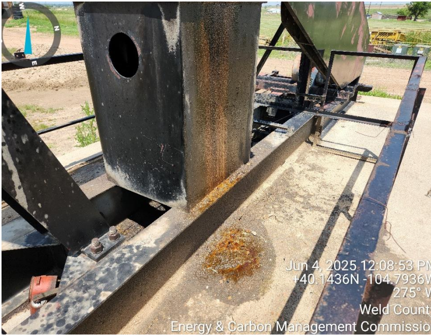
Photo 3 leak on pump jack gear box east side
