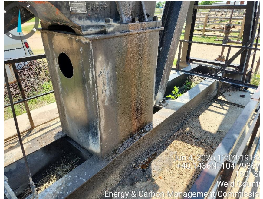
Photo 4 leak on pump jack gear box west side
