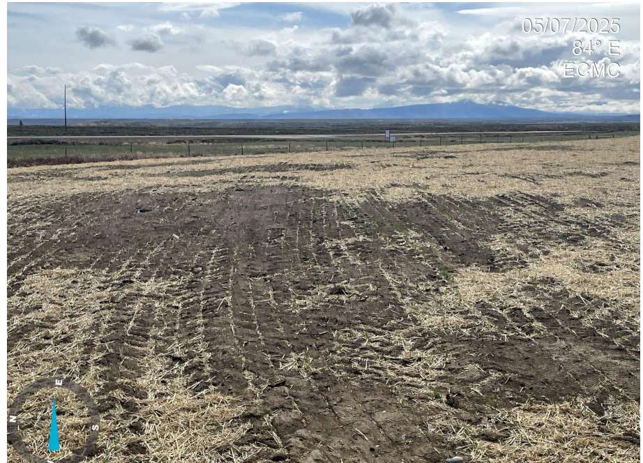
Photo 4. Photo taken from the northeastern portion of the pad, facing the eastern interim reclamation area. Photo illustrates seeding has occurred and straw mulch has been applied. Observed are areas where mulch does not appear to have been sufficiently anchored and has blown off.
