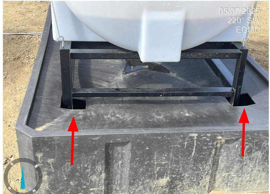
Photo 8. Photo taken from southeastern portion of Location of the tanks. Photo illustrates an example of missing caps/covers that prevent access to wildlife.
