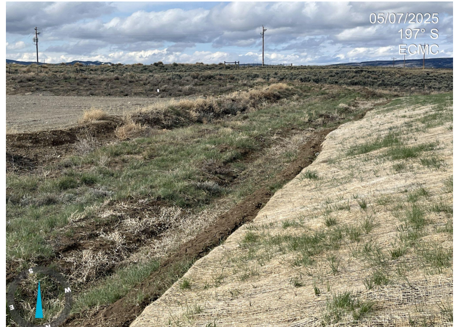
Photo 6. Photo taken from western portion of the location, facing south towards stockpiled soil. Erosion matting has been applied to soil stockpile.
