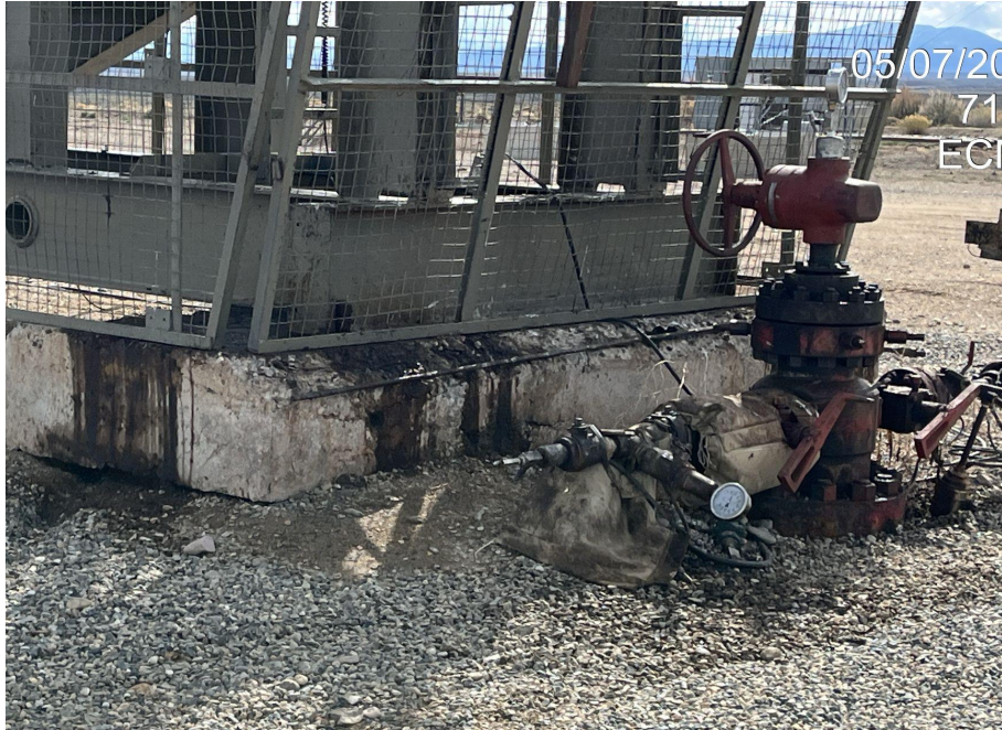
Photo 5. Photos 5-6 taken at the southwestern and eastern sides of the wellhead. Photos illustrates stained soils. Clean up soils pursuant to Rule 912 and maintain equipment per 608.e.
