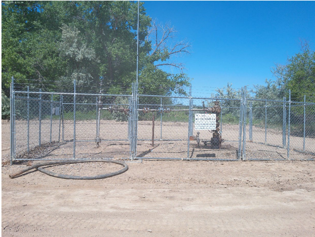
Injection Well head
